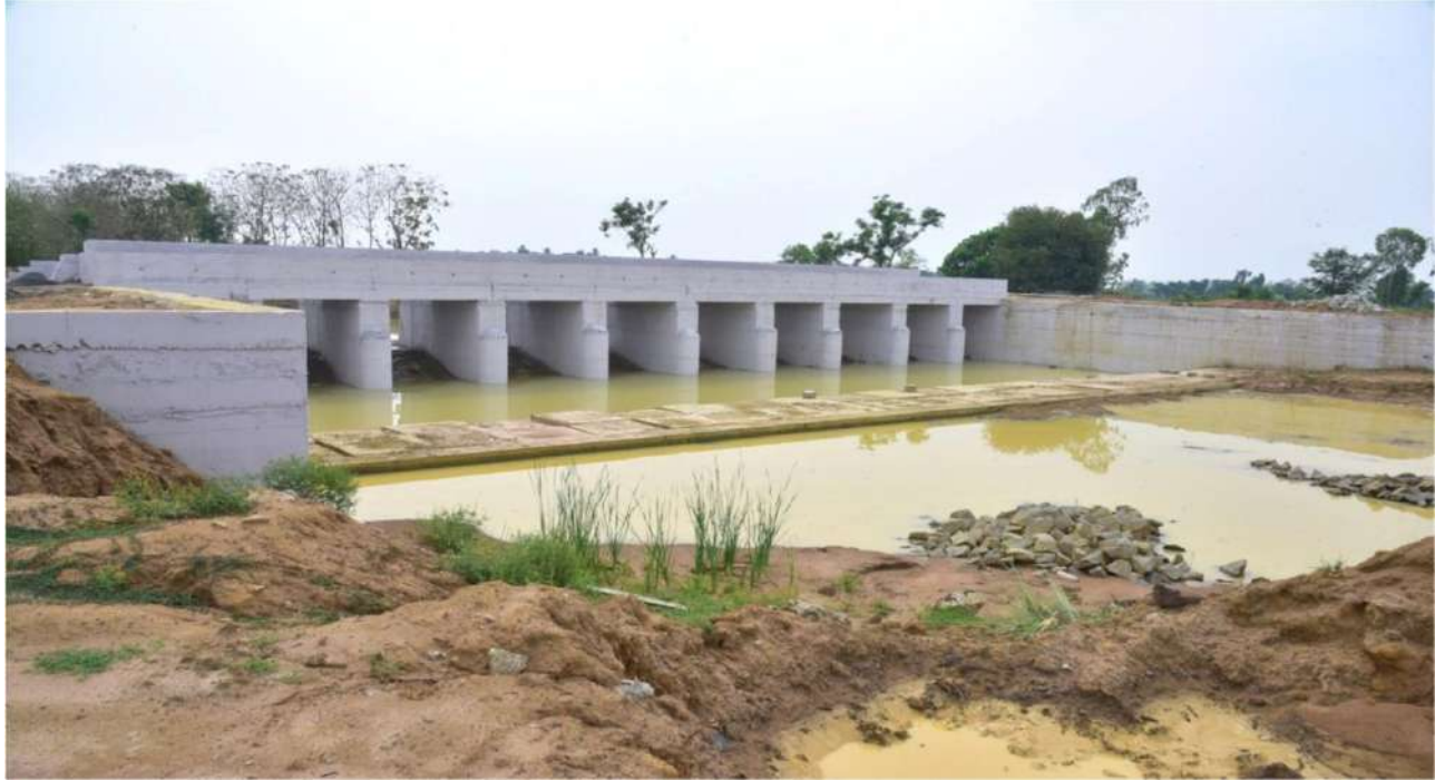
Cuddalore District – Kattumannar Koil Taluk– Sengal Odai – I – Regulator Rehabilitation work- TNIAMP Phase –II (package-I)- Veeranam Tank – Estimate Amount: Rs.55.05 Crore
