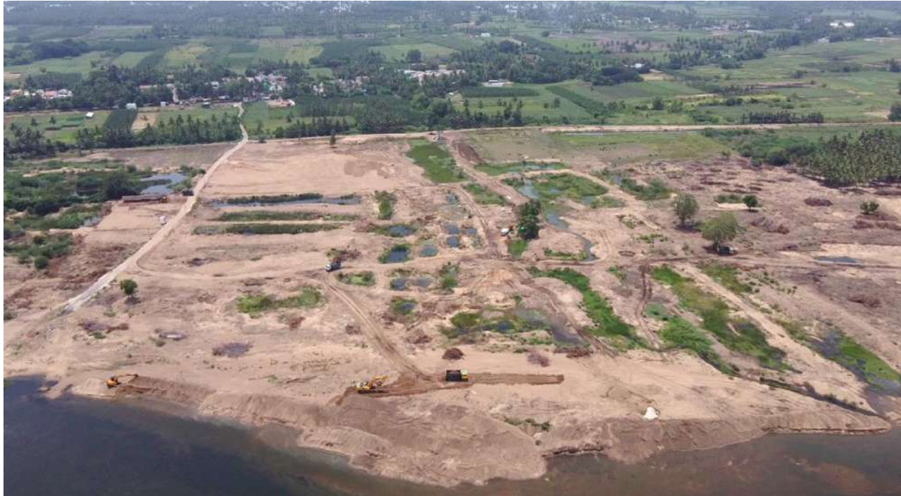
Karur District - Pugalur Taluk - Construction of Barrage across River Cauvery in Nanjai Pugalur Village Estimate Amount: Rs.406.50 Crore – Before
