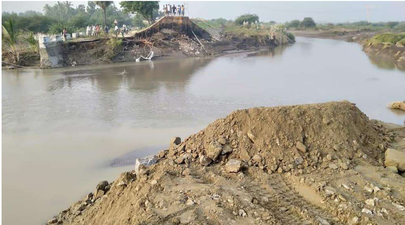
Thoothukudi District - Kalankarai Village -Temporary restoration to Tank bund breached in Korampallam Tank for a length of 132m - Before
