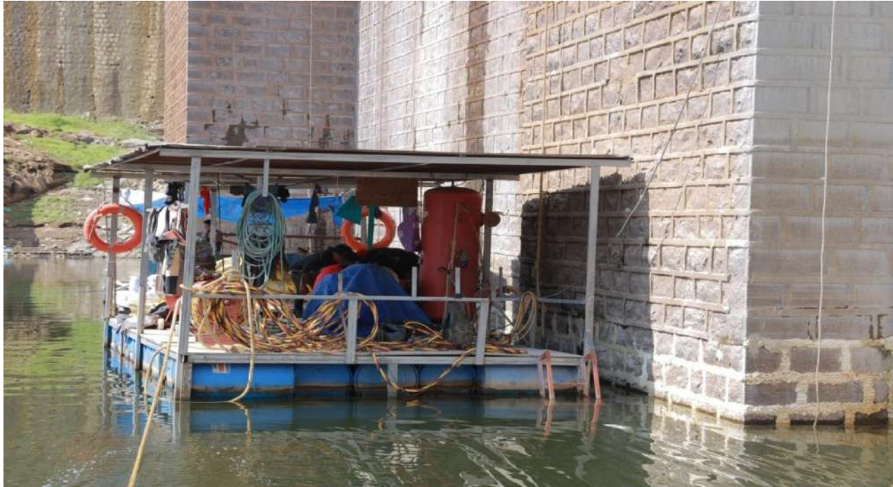
Coimbatore District - Valparai Taluk - Rehabilitation and improvement of Sholayar Dam - DRIP- Phase II (Racking and pointing in upstream face RR Joints at under water) - Estimate Amount : Rs.106.30 Crore
