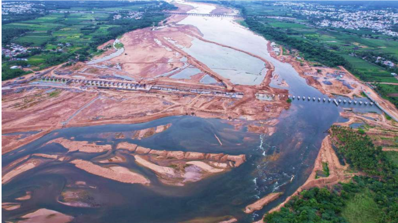
Karur District - Pugalur Taluk - Construction of Barrage across River Cauvery in Nanjai Pugalur Village Estimate Amount: Rs.406.50 Crore – Present Stage
