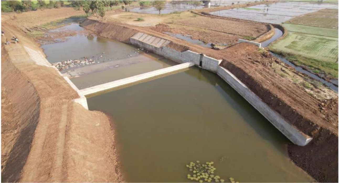
Viluppuram District & Taluk- Mandagapattu Village - Renovation of Mandagapattu Anicut across the Chellangal Odai - Estimate Amount:Rs.4.27 Crore
