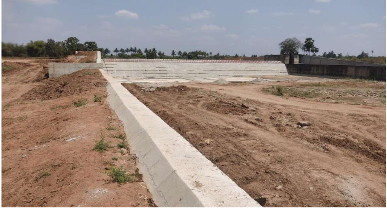
Viluppuram District - Vikkiravandi Taluk - V.Mathur Village - Renovation of V.Mathur Anicut across Pambai Channel- Estimate Amount : Rs.6.64 Crore
