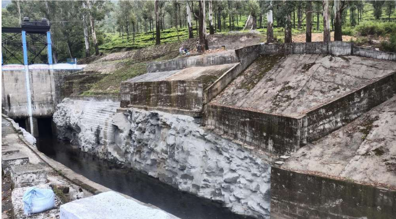
Coimbatore District - Valparai Taluk - Rehabilitation and Improvements to Upper Nirar weir (Tunnel Leading Channel Shotcrete Work)- Estimate Amount : Rs. 14.55 Crore
