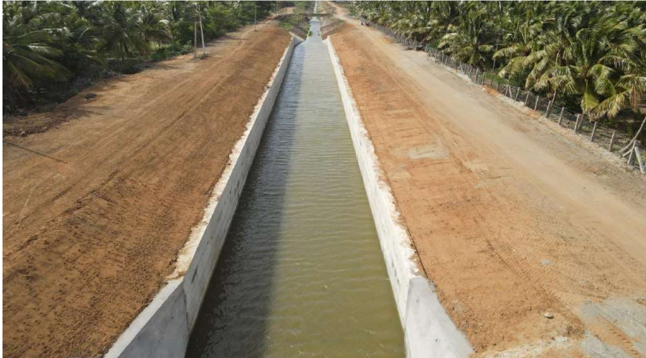
Tiruppur District, Udumalpet Taluk - Rehabilitation of Parambikulam Main Canal from L.S 3.000 km To 3.300 km – Estimate Amount Rs. 5.46 Crore
