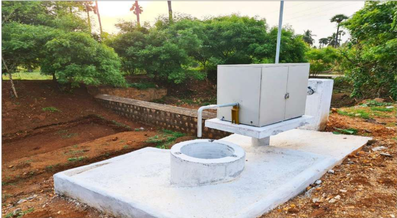
Erode, Coimbatore and Tiruppur District - Athikadavu Avinashi Pumping Scheme, Outlet Management System (OMS) in Pond - Estimate Amount Rs.1916.417 Crore
