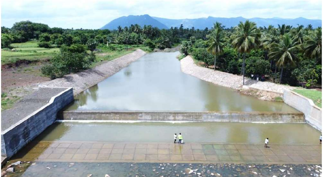
Tirupathur District - Tirupathur Taluk - Construction of Check dam across the Pambar river near Jondrampalli Village – Estimate Amount : Rs 3.33 Crore
