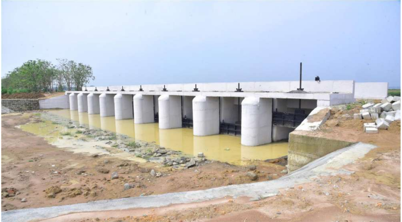
Cuddalore District – Kattumannar Koil Taluk - Andipalayam Regulator Rehabilitation work- Veeranam Tank – TNIAMP Phase –II (package-I) Estimate Amount: Rs.55.05 Crore
