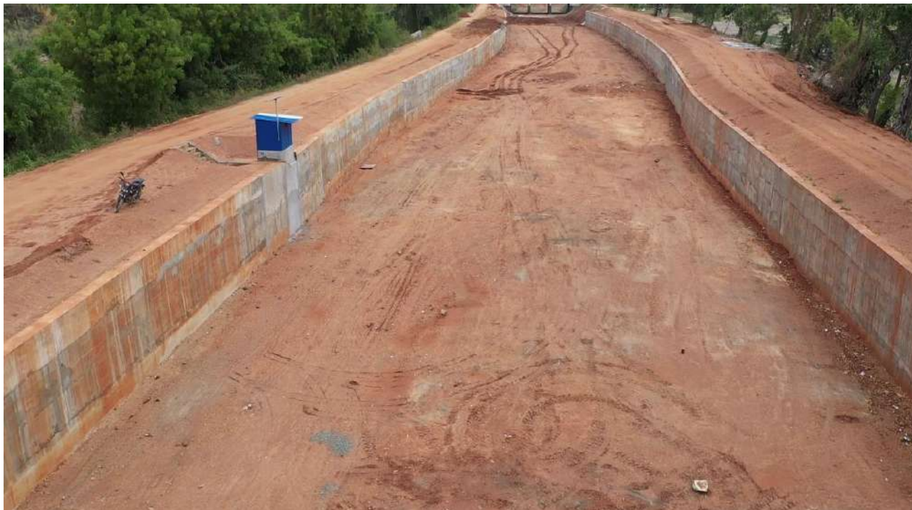
Erode, Tiruppur and Karur District – Extension, Renovation and Modernisation - Protection wall at Mile 53/3 in LBP Main Canal (Package no – 3) Estimate Amount - Rs.197.75 Crore
