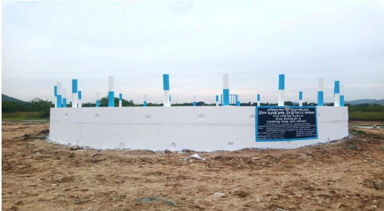
Thiruvallur District - Construction of 2 Nos of Artificial Recharge well Structures in Nandhiyar Sub basin – TNIAMP-II - Thadur Big Tank - Estimate Amount: Rs.91.90 lakh
