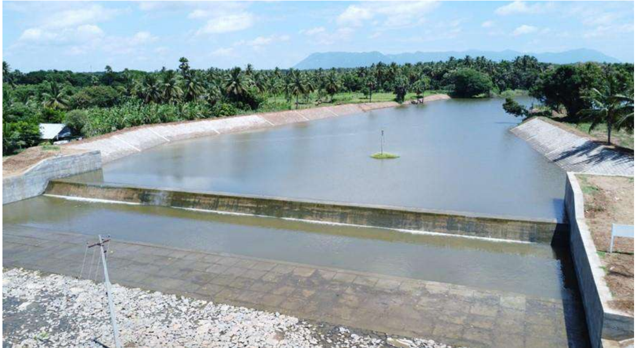
Tirupathur District - Tirupathur Taluk - Construction of Check Dam across Pambar River near Matrapalli Village - Estimate Amount : 3.80 Crore
