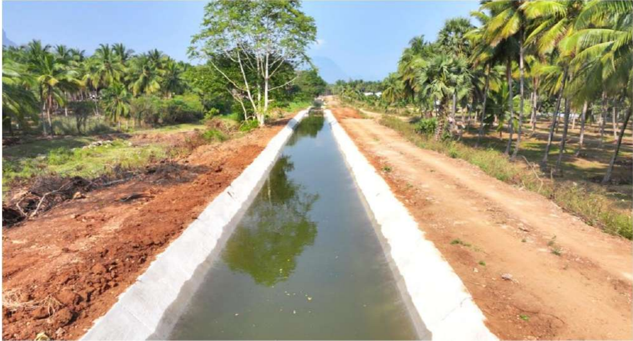
Coimbatore District, Anaimalai Taluk - Rehabilitation and Modernisation of Kulapathukulam Tank, 5 nos Anicuts & Anicut Channels and Vettaikaranpudur Canal and its Distributaries of Aliyar sub basin – Estimate Amount Rs. 34.19 Crore
