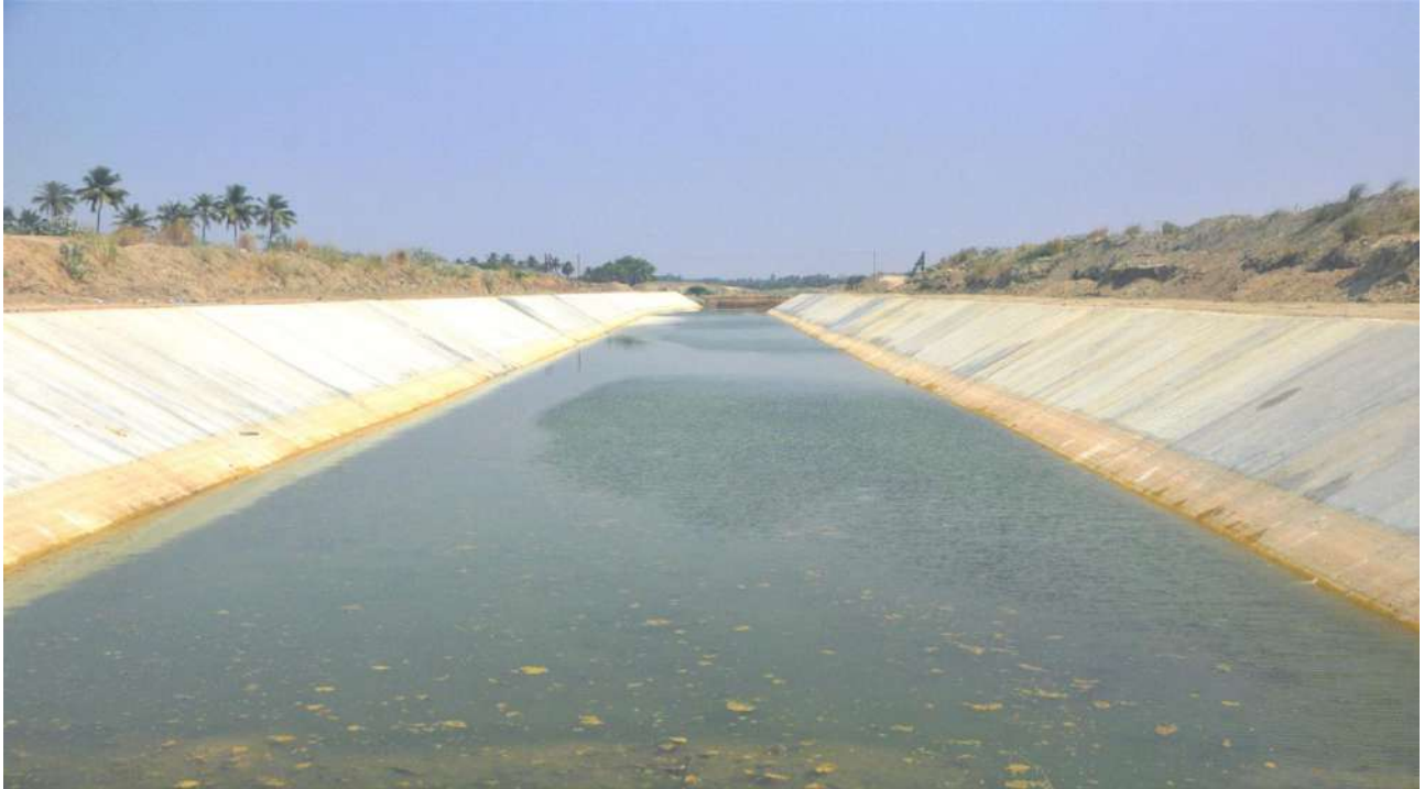
Karur District - Thirukampuliyur Village - Cauvery (Kattalai) – Vaigai – Gundar Flood Carrier Canal Project, Reach-1 of Slice-1 Canal lining at L.S 3800 m - Estimate Amount: Rs.177.03 Crore - After
