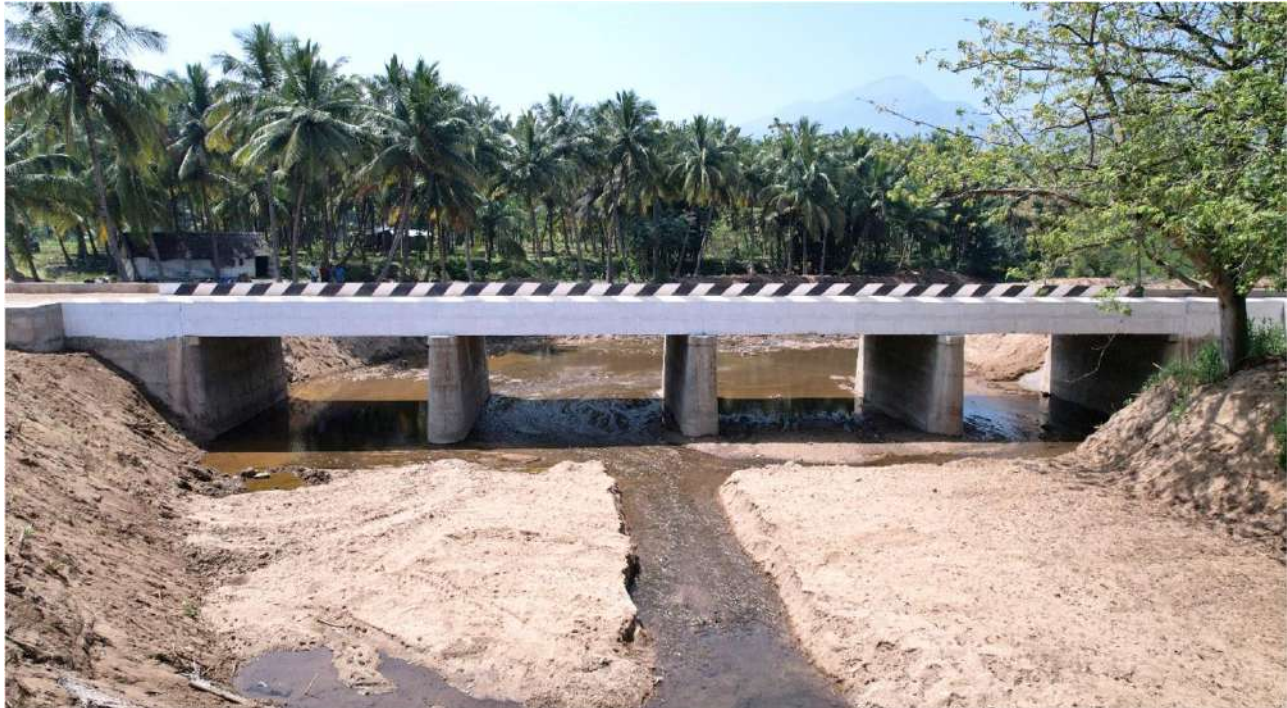
Virudhunagar District - Watrap Taluk - S.Kodikulam Village - Construction of Road Bridge across Kovilar River at LS 1600m - Estimate Amount: Rs.221.79 Lakh
