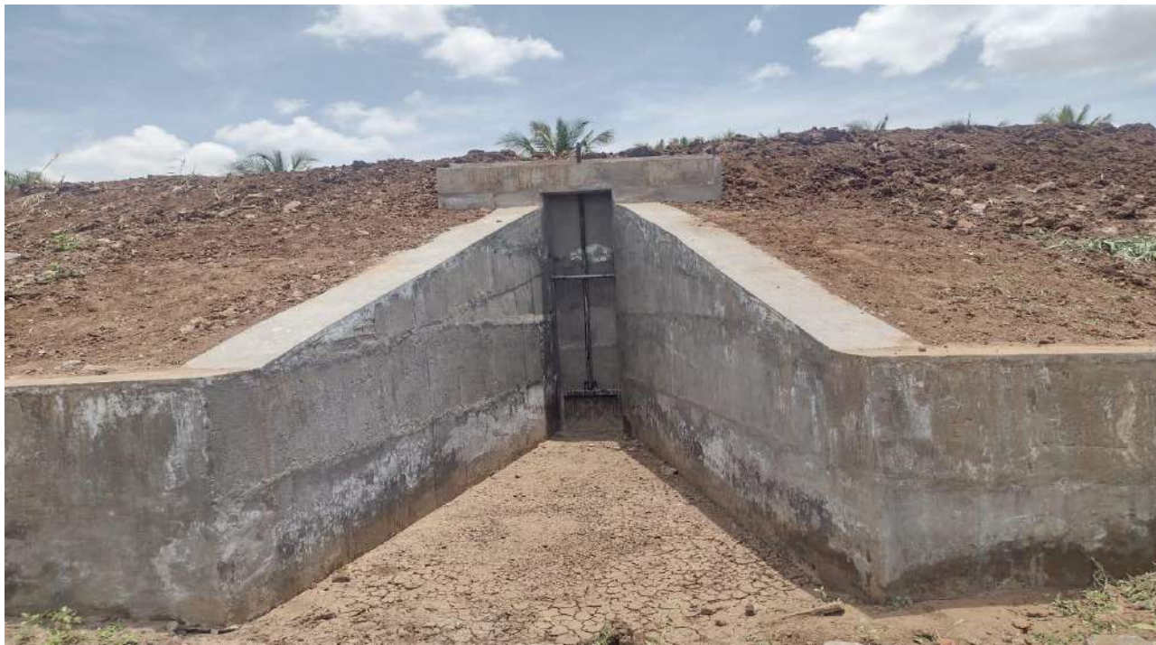
Dindigul District - Authoor and Natham Taluks & Blocks - Repair, Renovation and Restoration of 9 Tanks - RRR Phase V Scheme- Estimate Amount: Rs.4.23Crore
