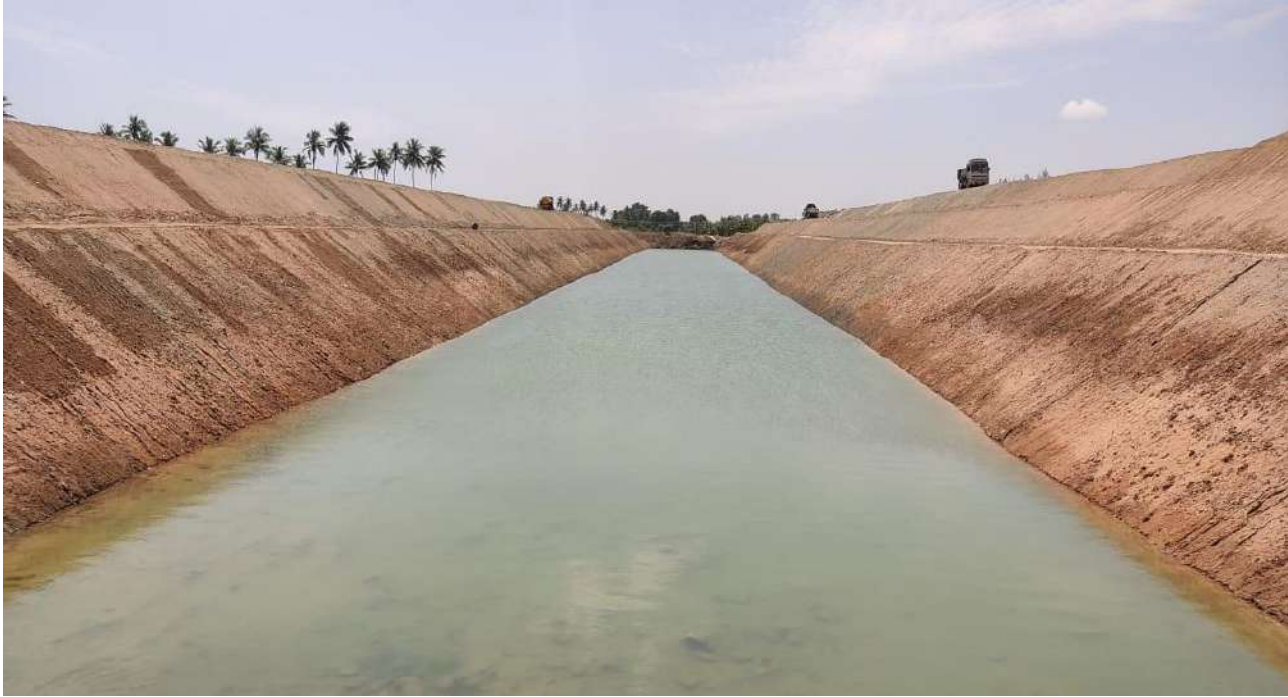
Karur District - Thirukampuliyur Village - Cauvery (Kattalai) – Vaigai – Gundar Flood Carrier Canal Project, Reach-1 of Slice-1 Canal lining at L.S 3800 m - Estimate Amount: Rs.177.03 Crore - Before
