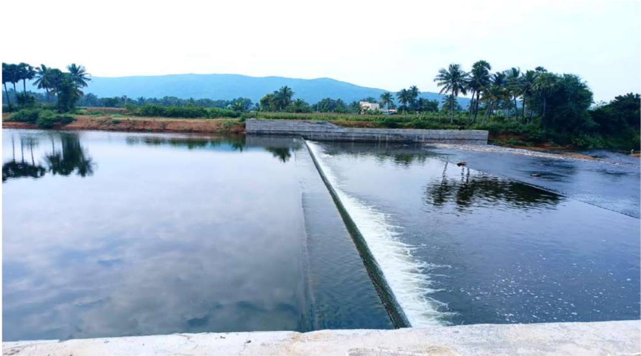
Salem District - Gangavalli Taluk - Gangavalli Village - Construction of Checkdam across Swetha nadhi at Kanavai Kadu in - Estimate Amount : Rs. 3.80 crore
