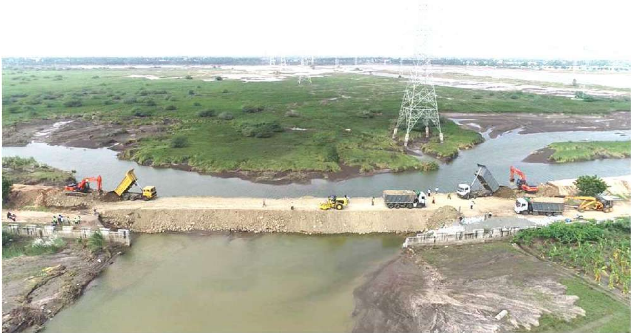
Thoothukudi District - Kalankarai Village -Temporary restoration to Tank bund breached in Korampallam Tank for a length of 132m - After
