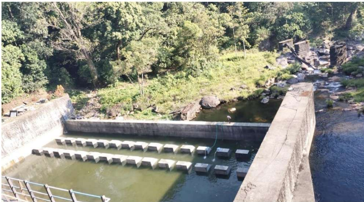
Coimbatore District – Valparai Taluk – Rehabilitation and improvement of Upper Nirar weir DRIP- Phase II (Stilling Basin ) – Estimate Amount : Rs.14.55 Crore
