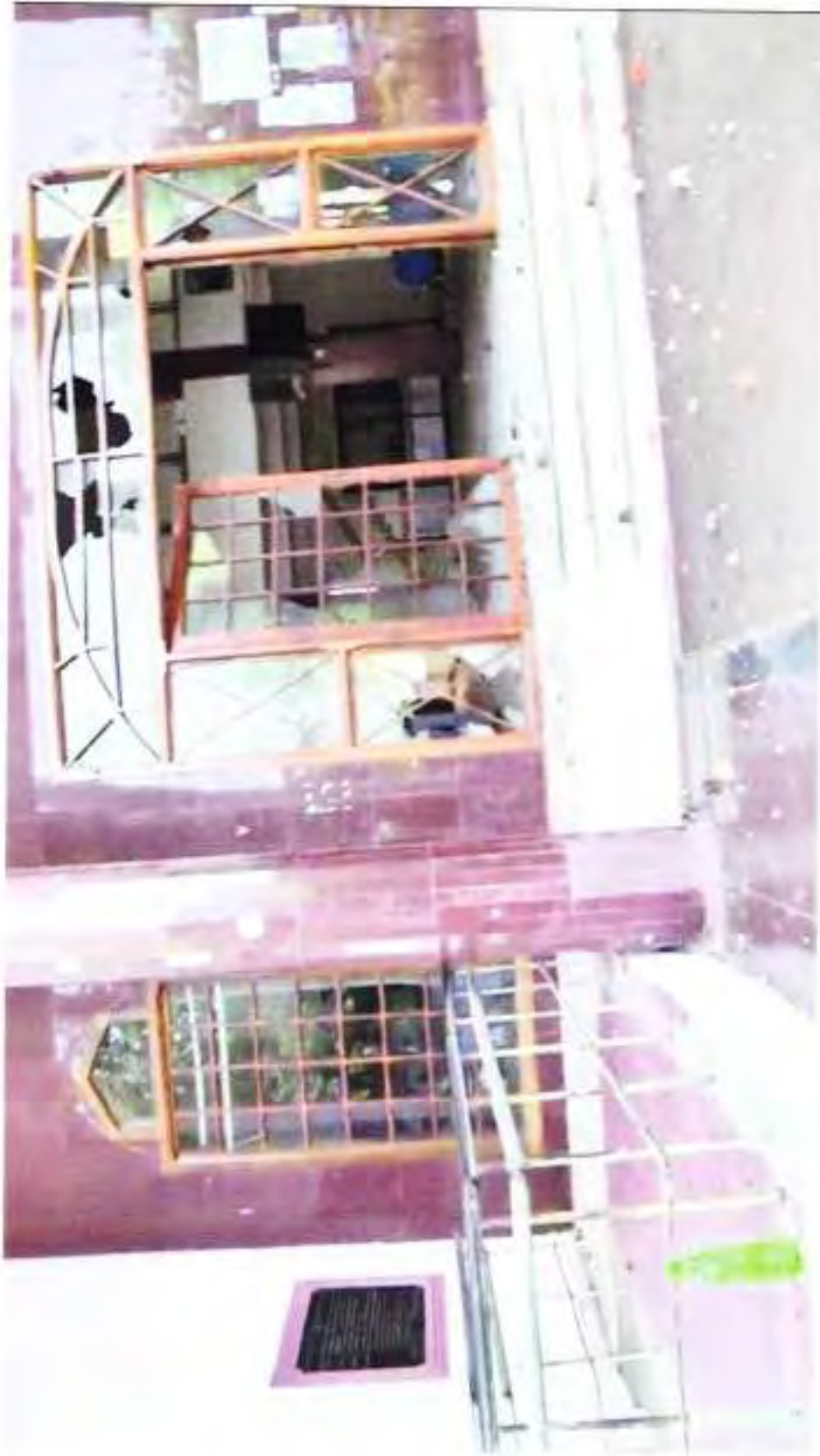
COLLECTOR OFFICE DAMAGE
