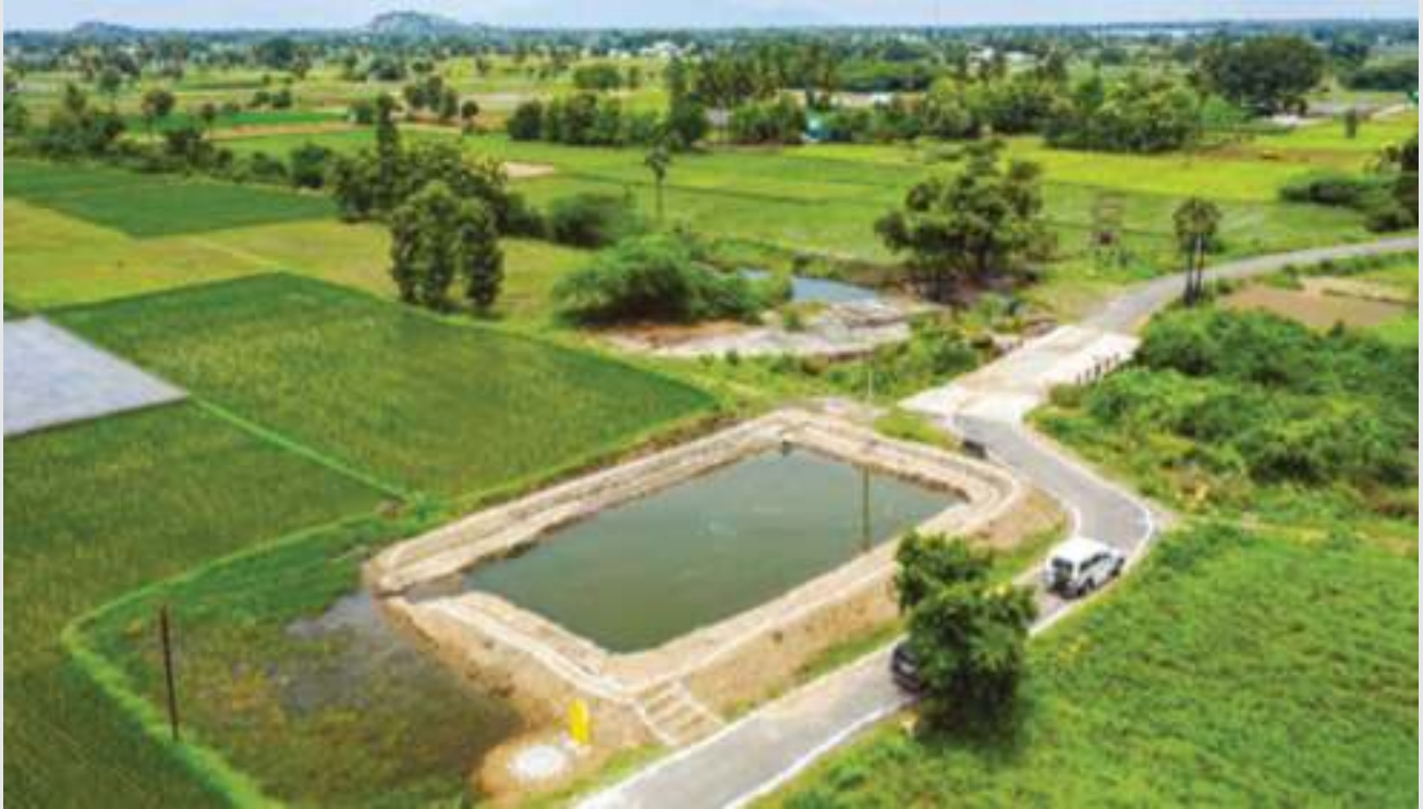
Construction of Farm pond in Seelapandal Panchayat in Thurinjapuram Panchayat Union of Tiruvannamalai District under Mahatma Gandhi National Rural Employment Guarantee Scheme at an estimate of Rs.1.78 lakhs
