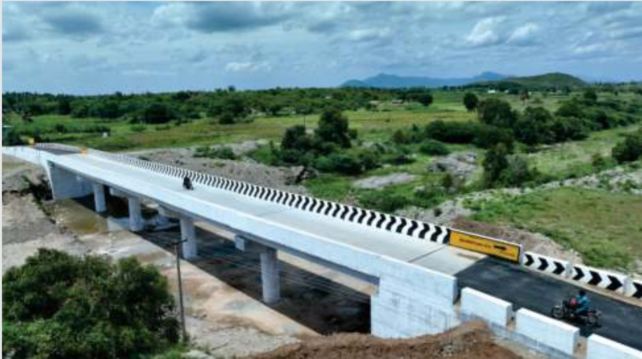
Construction of Bridge across Vaniar River at Km 1/6 of Sattaiampatti to Kailavaram road in Harur Panchayat Union of Dharmapuri District under NABARD RIDF at an estimate of Rs. 395.46 Lakh
