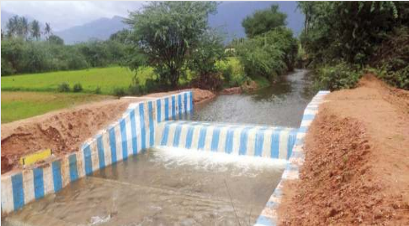
Construction of Check Dam across Veeraiyan Odai in Melachinthalaichery Panchayat of Uthamapalayam Panchayat Union of Theni District under Mahatma Gandhi National Rural Employment Guarantee Scheme at an estimate of Rs.7.40 lakhs
