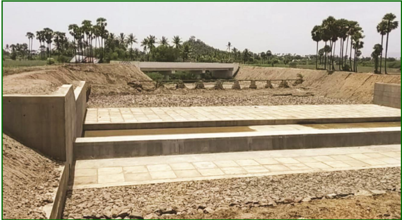
Salem District – Check Dam constructed across Sarabanga River in Dadarapuram Village (Estimate Amount Rs.2.58 crore)
