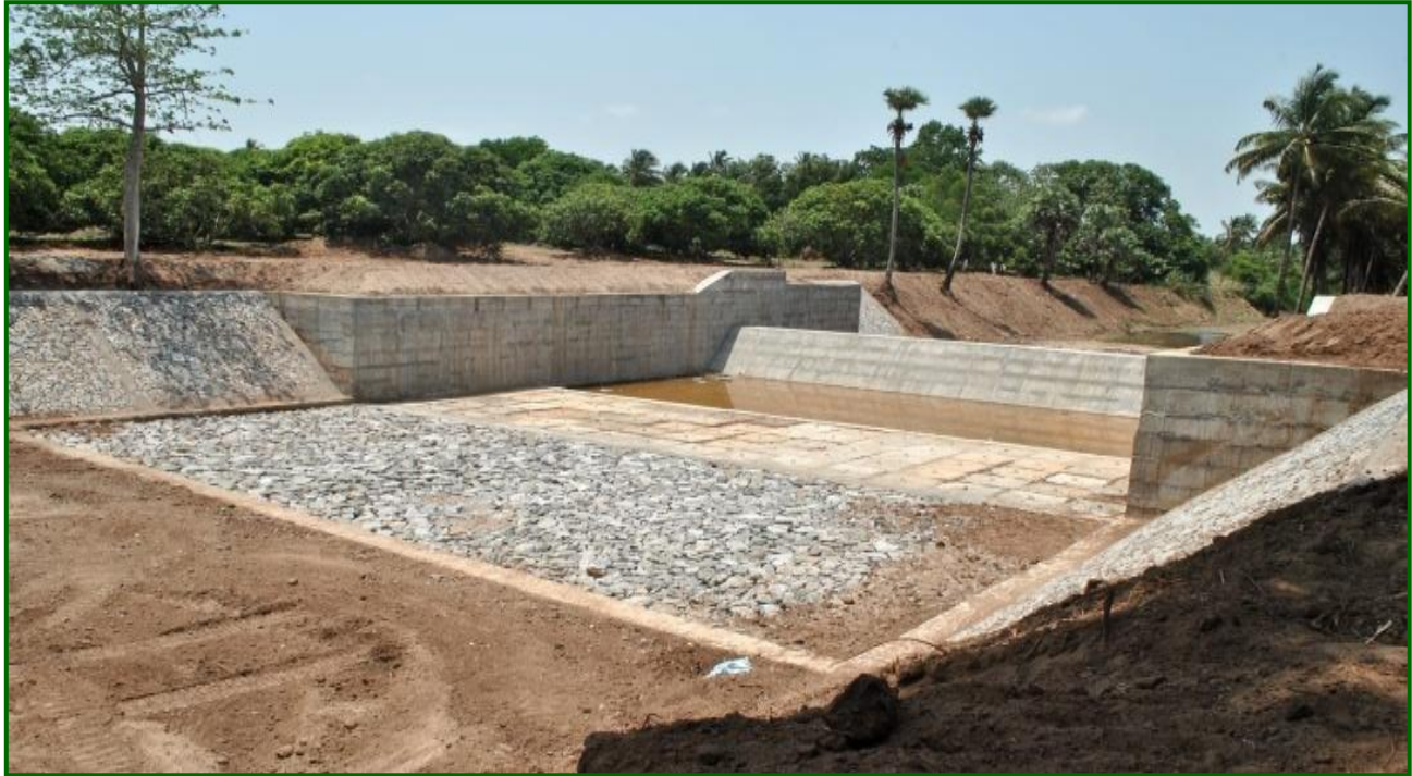
Coimbatore District – Construction of Check Dam across Korai River in Mannur Village of Pollachi Taluk (Estimate Amount: Rs.90.00 Lakh)
