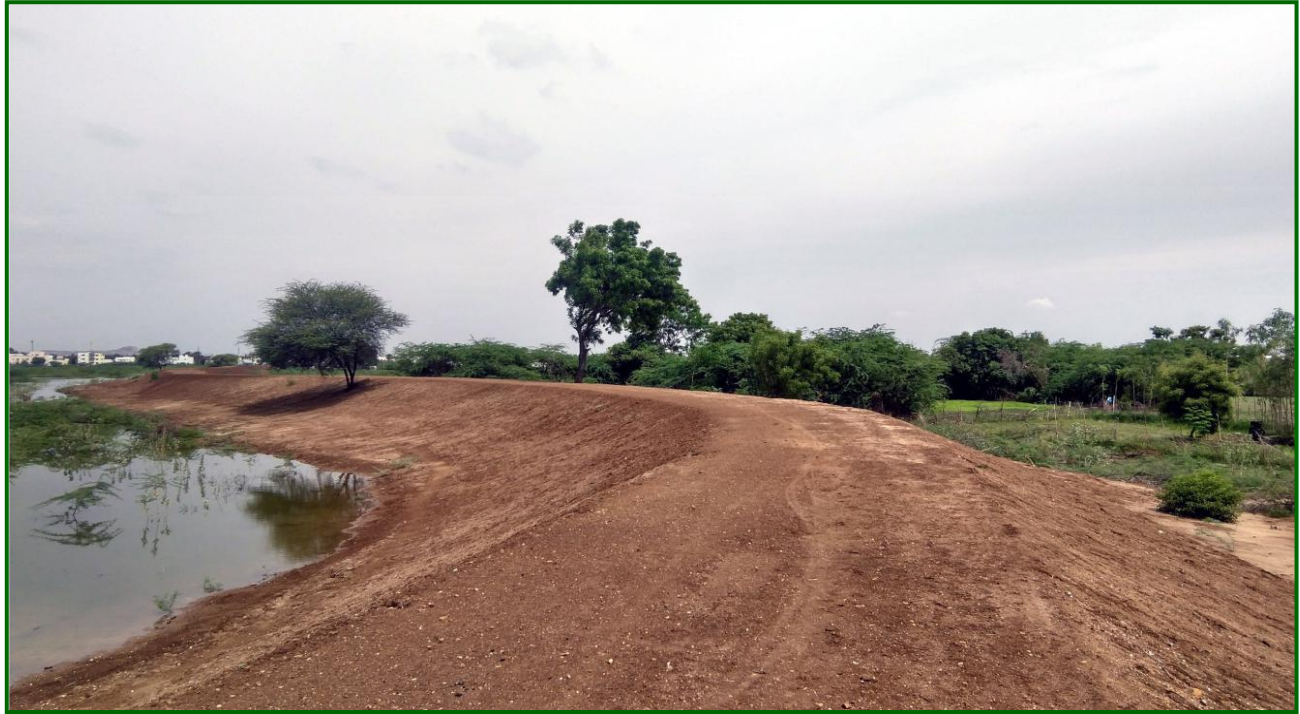
Madurai District – Rehabilitated Anaiyur Tank in Anaiyur Village (Estimate Amount Rs.3.27 crore)
