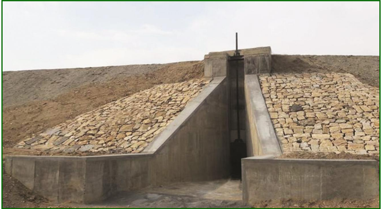
Salem District – Rehabilitated Achampalli Tank Sluice in Konganapuram Village (Estimate Amount Rs.0.10 crore)
