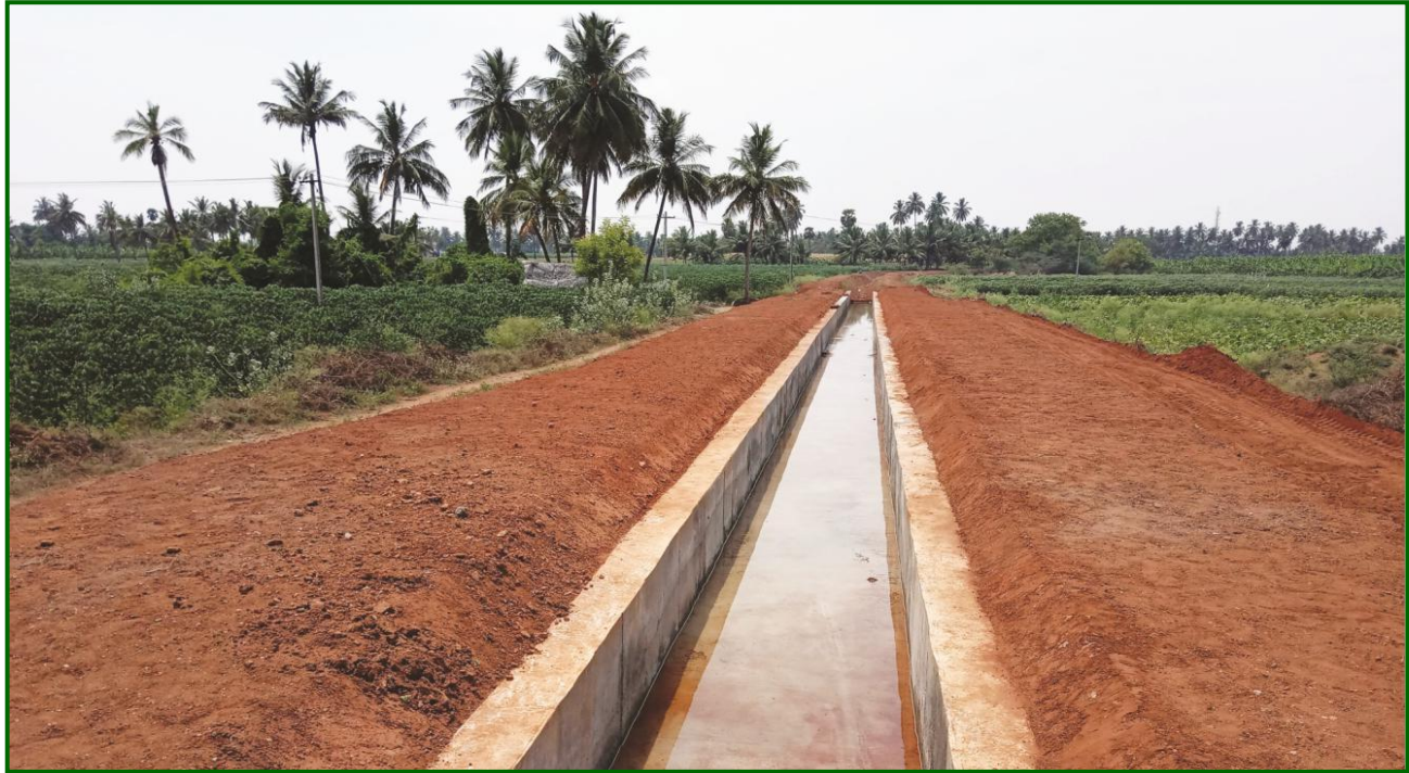
Erode District – Rehabilitated Elathur Anicut Channel in Elathur Village (Estimate Amount Rs.1.97 crore)
