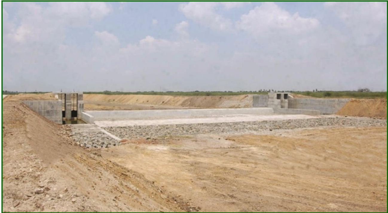
Virudhunagar District – Anicut constructed across Kowsikanadhi to feed Kalaperumalpatti Tank in Avudayapuram Village (Estimate Amount Rs.3.50 crore)
