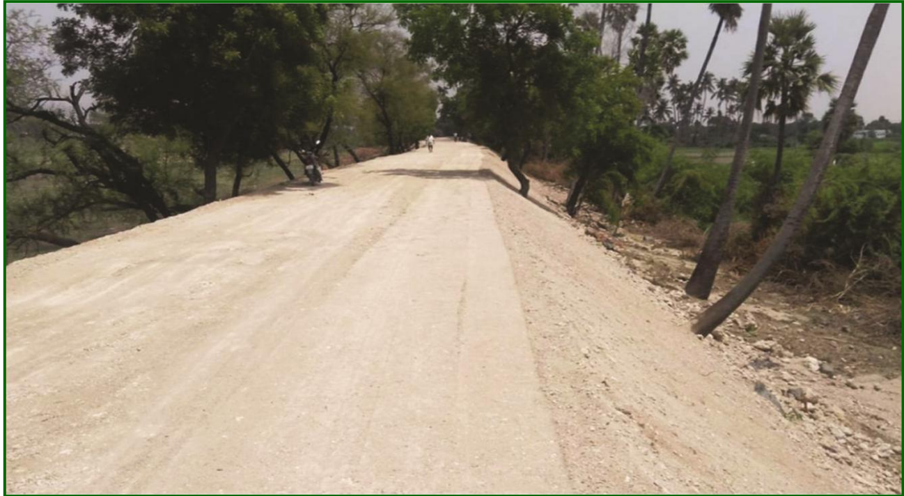
Salem District – Rehabilitated Deviyakurichi Tank in Deviyakurichi Village (Estimate Amount Rs.0.295 crore)
