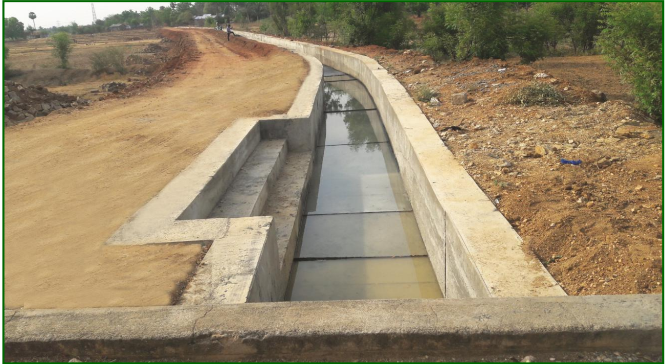
Erode District – Rehabilitated Nallampatti Anicut Channel in Nallampatti Village (Estimate Amount Rs.0.59 crore)
