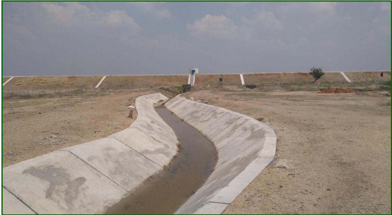
Virudhunagar District – Rehabilitated Main Canal of Kullursandai Rservoir in Aruppukottai Taluk (Estimate Amount Rs.2.54 crore)
