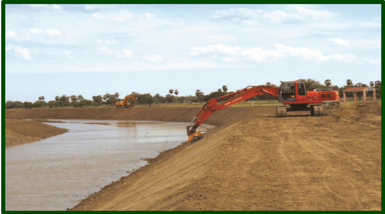
Nagapattinam District - Strengthening of Pandavayar River Bund in Killkudi Village under ADB assistance
