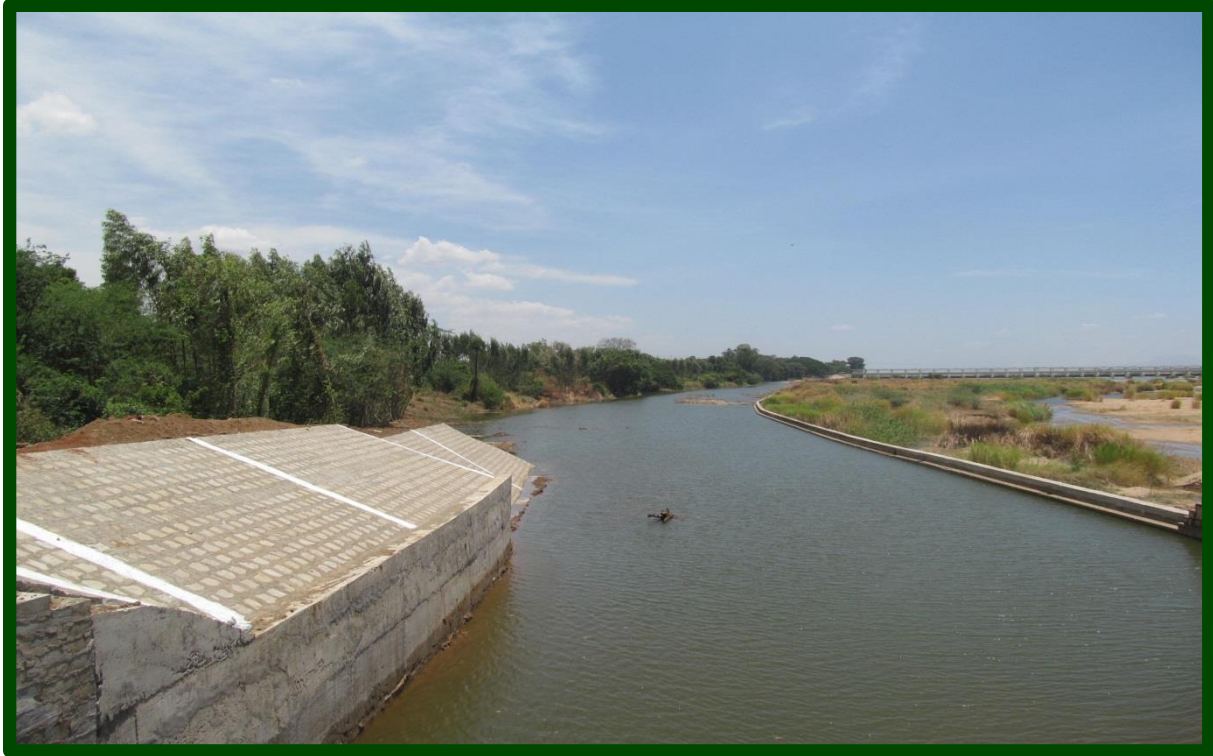
Trichy District - Protection of Right Bank of River Cauvery at Downstream of Upper Anicut in Srirangam Taluk
