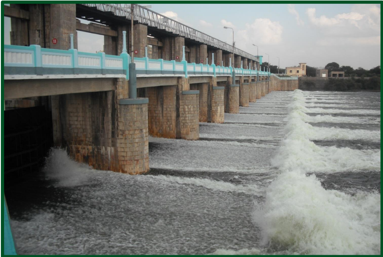
View of surplus discharge from the Saddle of Sathanur Dam, awarded as the best maintained dam for the year 2015-2016
