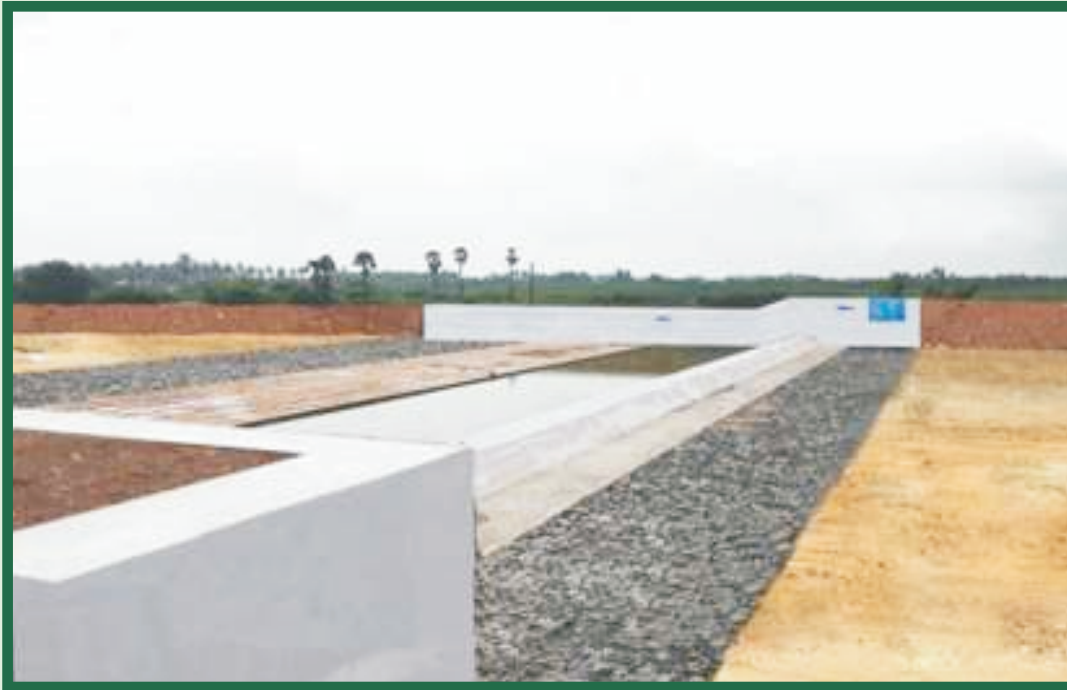
Check Dam Constructed across Karaipottanar River in Nagayanallur Village of Thottiyam Taluk in Trichy District under NABARD Scheme
