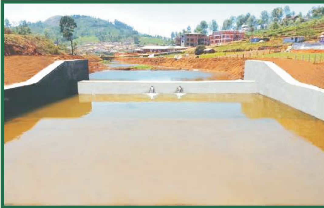
Check dam constructed near Millidane in Nedugula (kappatty) Village in Kothagiri Taluk of Nilgiris District under NABARD assistance
