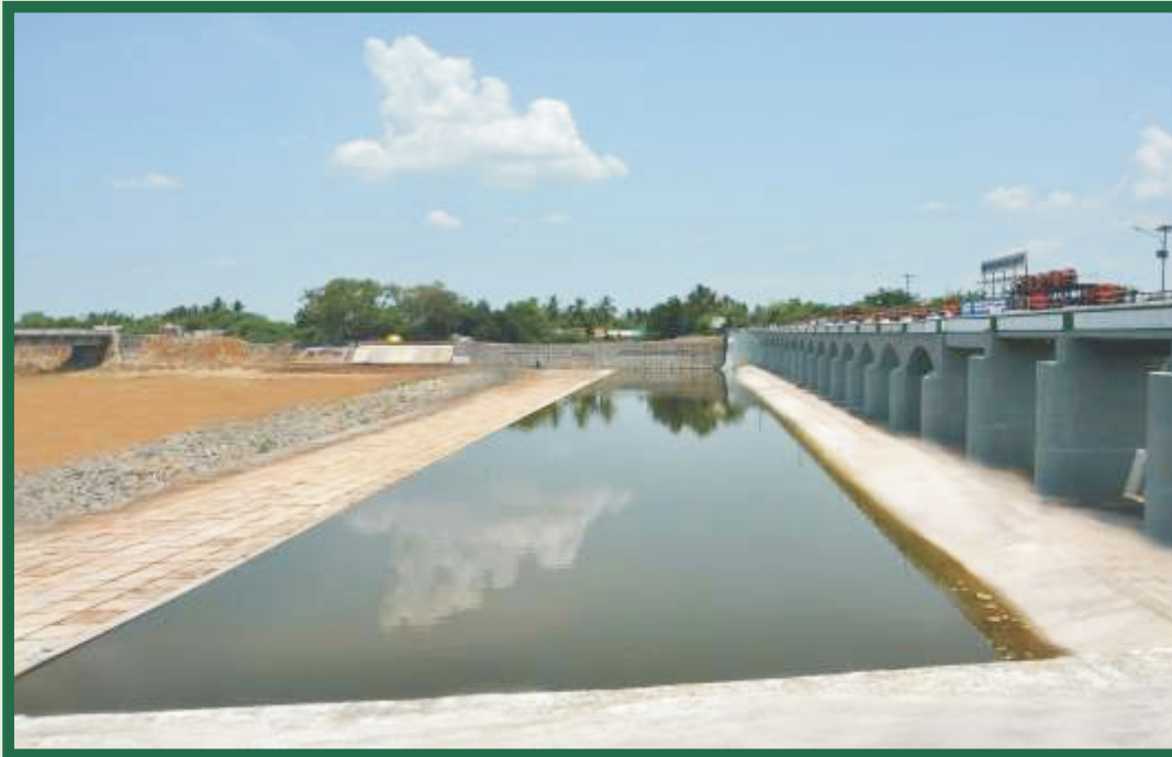
Rehabilitated Sethiathope (Regulator) Anicut across Vellar River in Chidambaram Taluk of Cuddalore District under NABARD Scheme
