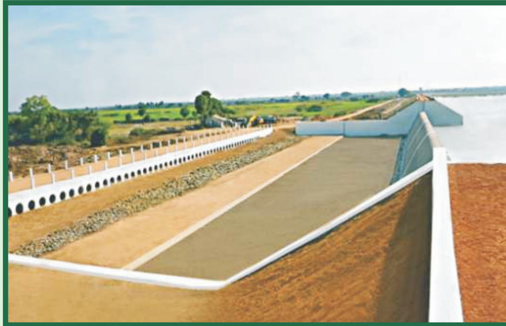
Rehabilitated and Improved Sidhamalli Dam in Karkudi Village of Udayarpalayam Taluk in Ariyalur District under Dam Rehabilitation and Improvement Project
