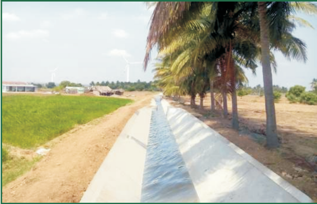
New Canal constructed for Linking of Parambikulam Aliyar Project system to Uppar Canals in Dharapuram Taluk of Tiruppur District under NABARD assistance
