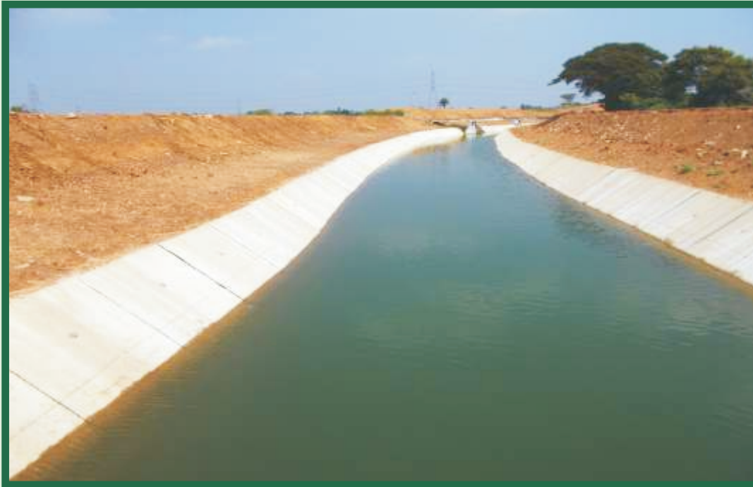
Strengthened slipped portion of Kandaleru Poondi canal at L.S.13.000 km to 25.275 km in Uthukottai Taluk of Tiruvallur District under NABARD Scheme
