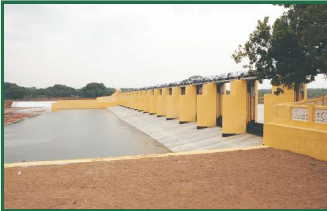
Rehabilitated Pelandurai Regulator across Vellar River in Thittagudi Taluk of Cuddalore District under NABARD Scheme
