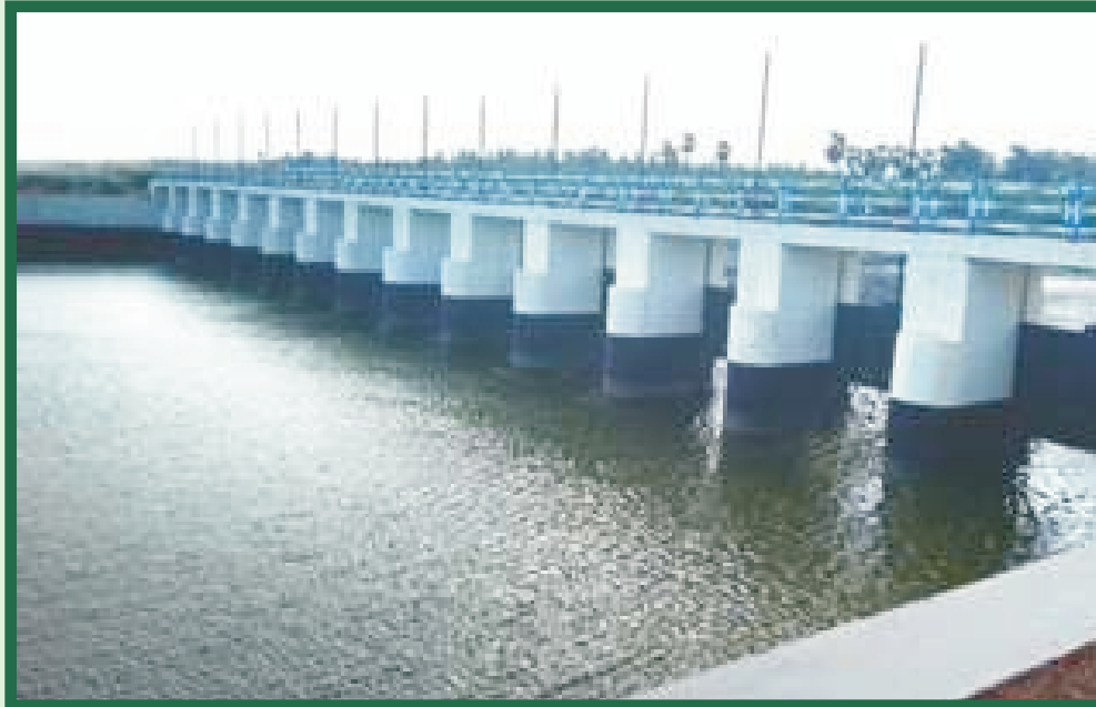
Tailend Regulator constructed across Kandaparichanar Drain at LS 26.400 km in Jambuvanodai Village of Thiruthuraipoondi Taluk in Thiruvarur District under NABARD Scheme
