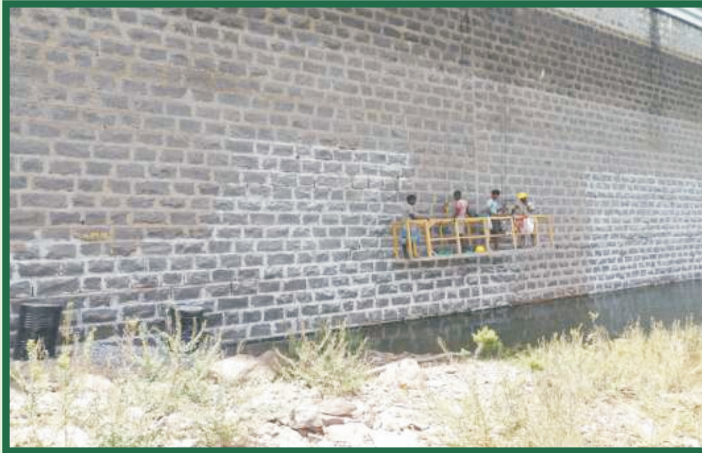
Rehabilitation of Aliyar Dam in Pollachi Taluk of Coimbatore District under Dam Rehabilitation and Improvement Project
