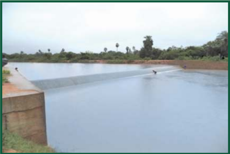
Check dam with Recharge shaft constructed across Nallodai near Sathipattu Village in Panruti Taluk of Cuddalore District under Master Plan Artificial Recharge Scheme
