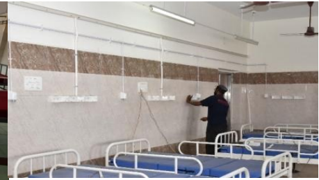
Additional beds with Medical Oxygen facilities at Government Hospital, Ponneri
