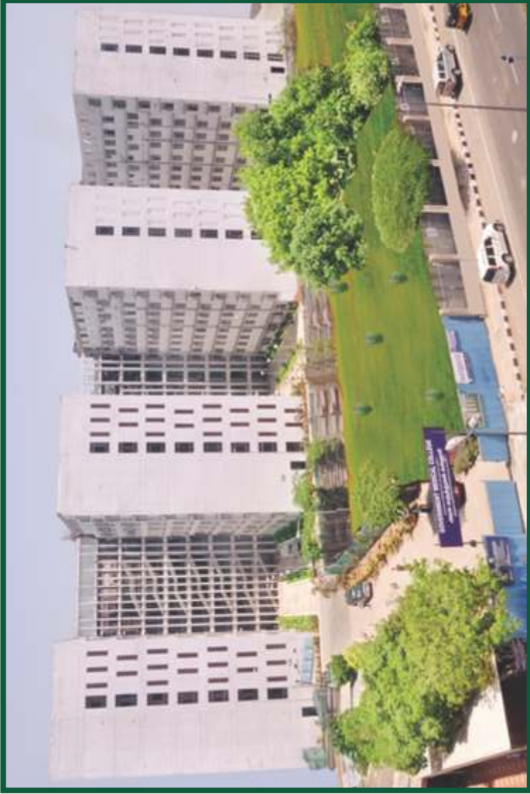
New Medical College and Hospital at Omandurar Government Estate Campus, Chennai Estimate Cost - Rs.123.30 Crore – Progress
