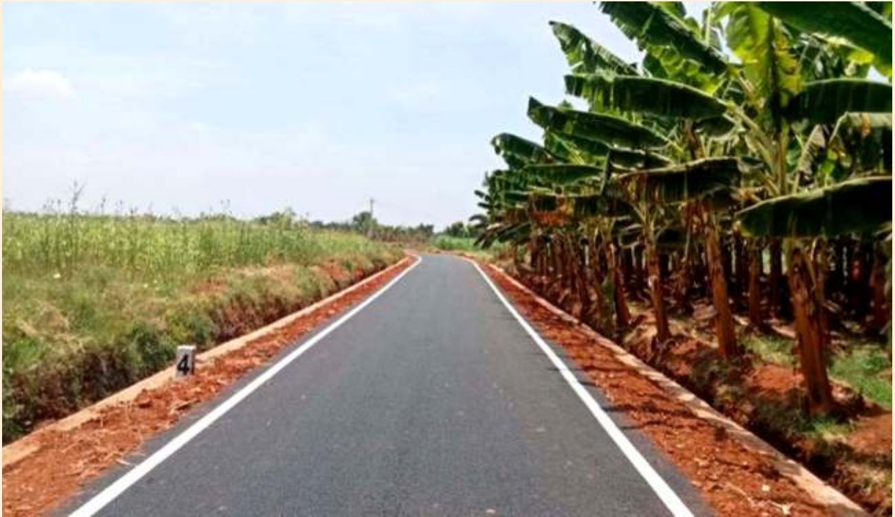
Construction of BT Road and Retaining wall at Valliyampalayam road, Vellankattupalayam in Lakkampatti Town Panchayat, Erode District. Estimate Cost: 1.22 Crore
