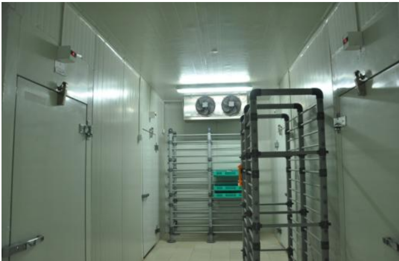
An inside view of Cold Chamber of Bivoltine Grainage at Krishnagiri
