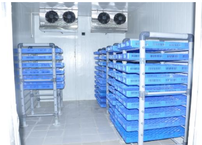
Inside View of Cold Chamber at Bivoltine Grainage of Krishnagiri.
