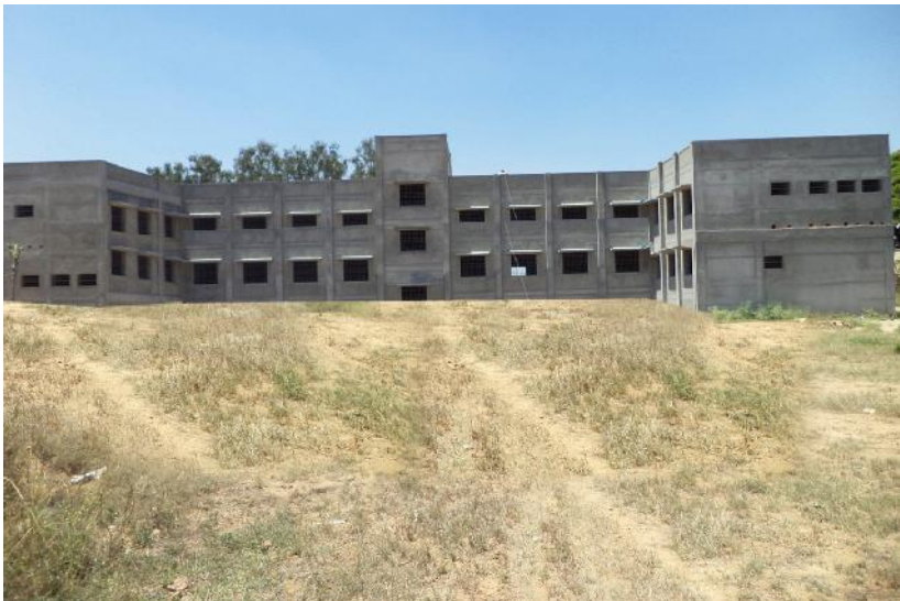
A View of the New Block being constructed at Tamil Nadu Sericulture Training Institute, Hosur
