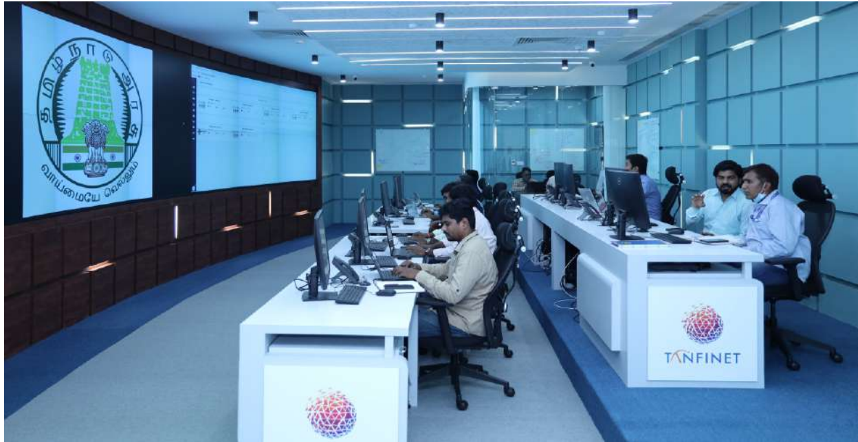
A State of Art Network Operation Center to monitor BharatNet Point of Presence (12525 Gram Panchayat & 388 Blocks) across the State was established at a cost of Rs.43.46 Crore in Chennai
