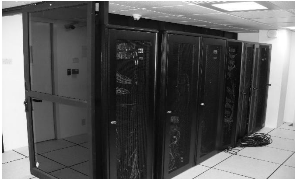
Figure 12: Cloud Infrastructure at TNSDC - 1
