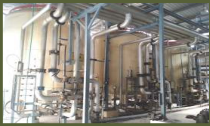
Filtration section at Arulpuram CETP
