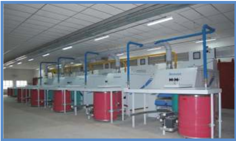
Carding section at Ramanathapuram Co-operative Spinning Mills
