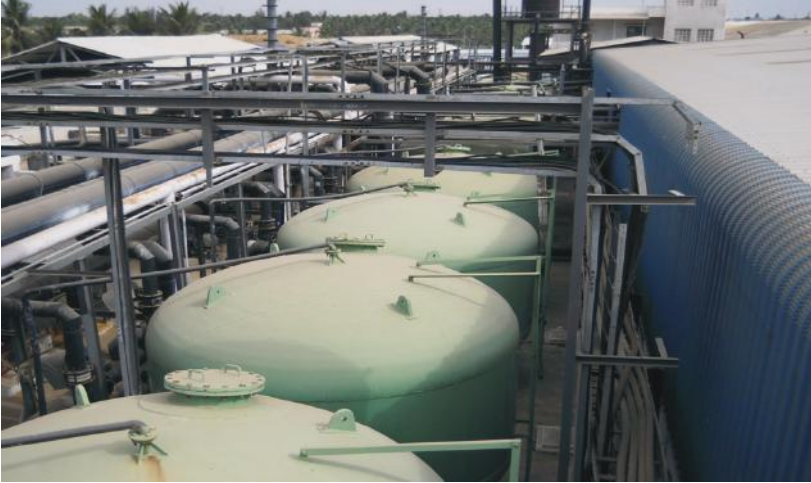
Dual Media Filter of Veerapandi Common Effluent Treatment Plant
