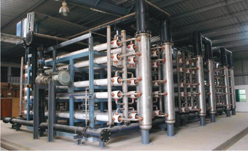
Ultra filtration Reverse Osmosis system of Veerapandi CETP
