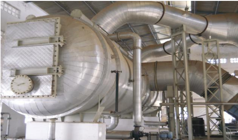
Mechanical Vapour Recompression (MVR) Plant of Sirupooluvapatti CETP
