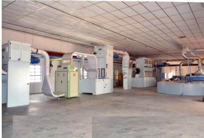
Bharathi Co-operative Spinning Mill Blow Room
