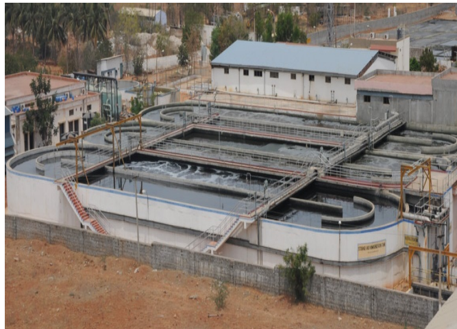
Common Effluent Treatment Plant, Tiruppur, Bio Filtering Section
