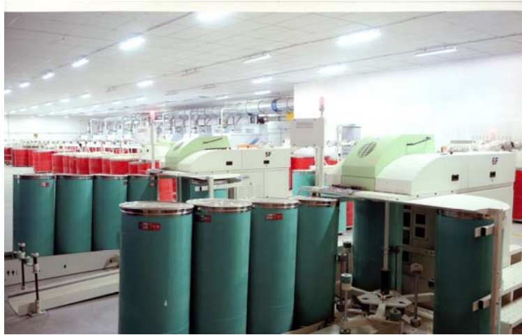
Pudukottai District Co-operative Spinning Mill Drawing Section
