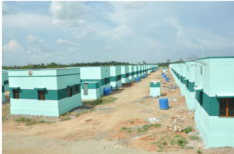
A Cluster of Green Houses under Construction at Tiruppur Block in Tiruppur District
