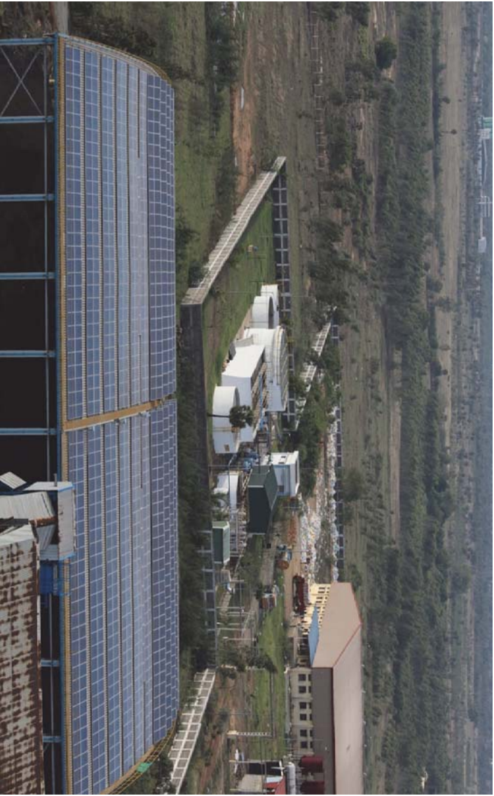
Roof Top Solar Panels in a Coal based Power Plant in Tiruvallur District
