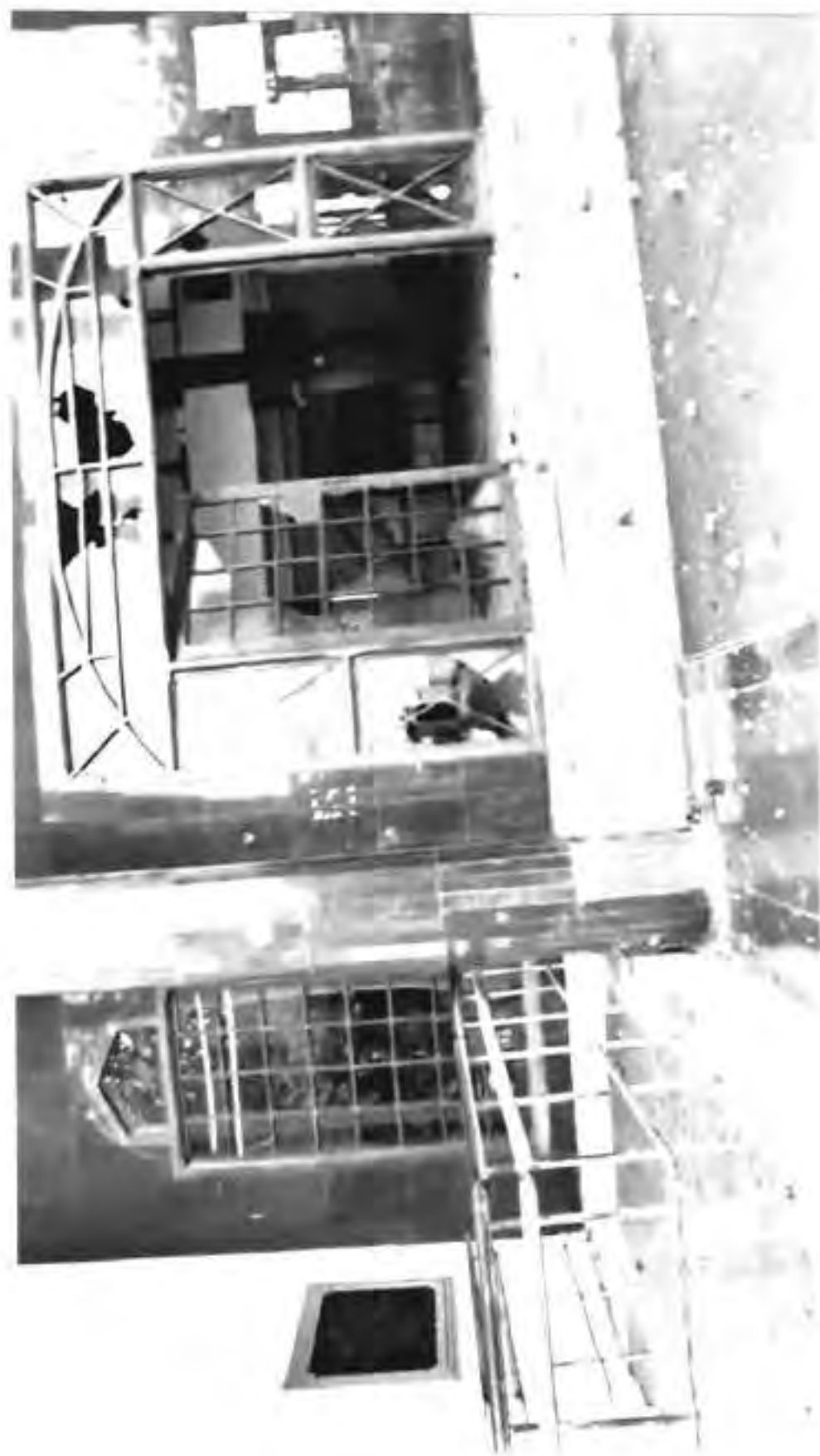
COLLECTOR OFFICE DAMAGE
