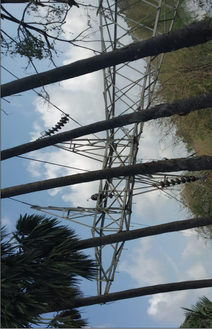
Damages Caused to Infrastructure due to GAJA Cyclone
