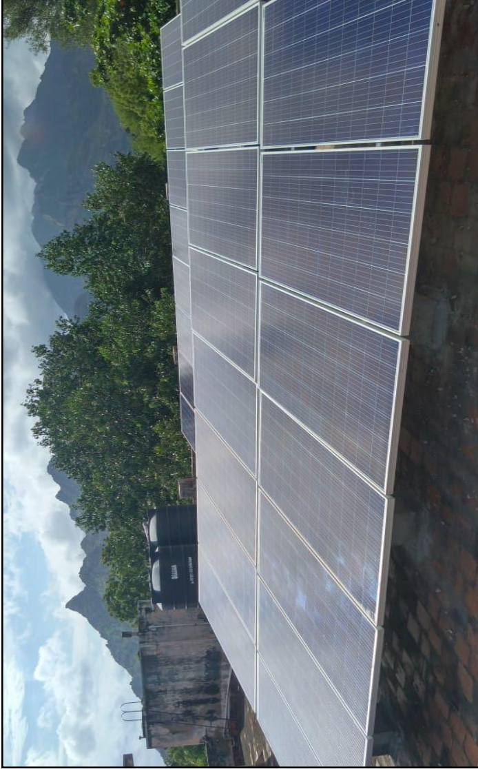
Two numbers 20 KW and 10 KW Solar Panels installed at Superintending Engineer/ Kanyakumari Electricity Distribution Circle
