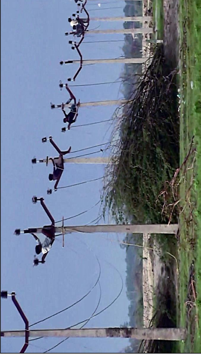
Damages Caused to Infrastructure due to GAJA Cyclone
