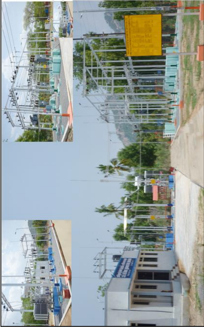
Modikuppam 33/11kV SS – Vellore District
