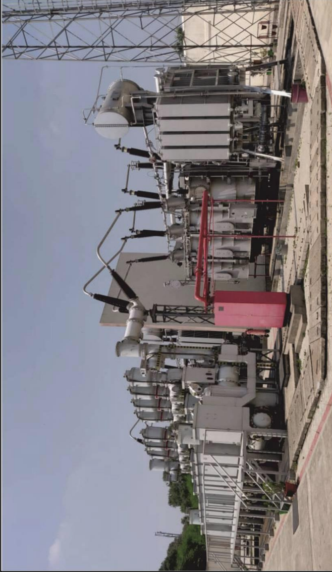
Central 230/110 kV GIS Sub Station, Chennai
