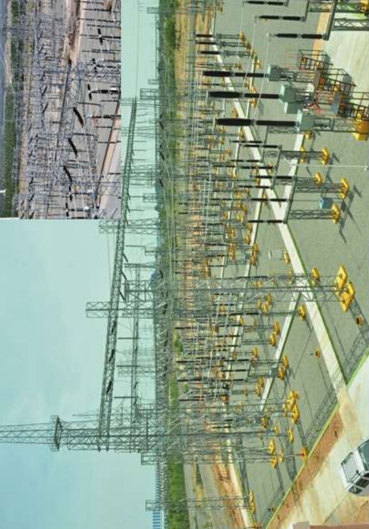
Annakadu 400/ 230-110kV Substation – Tiruppur District
