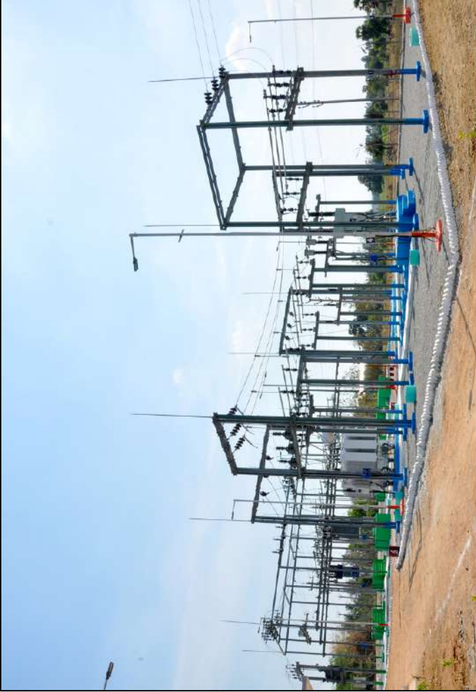
DDUGJY scheme- Melma 33/11 kV substation - Tiruvanamalai District
