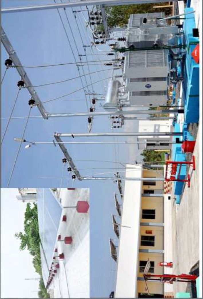
IPDS scheme- Makinamkombai 33/11kV Substation along with Solar roof top- Erode District
