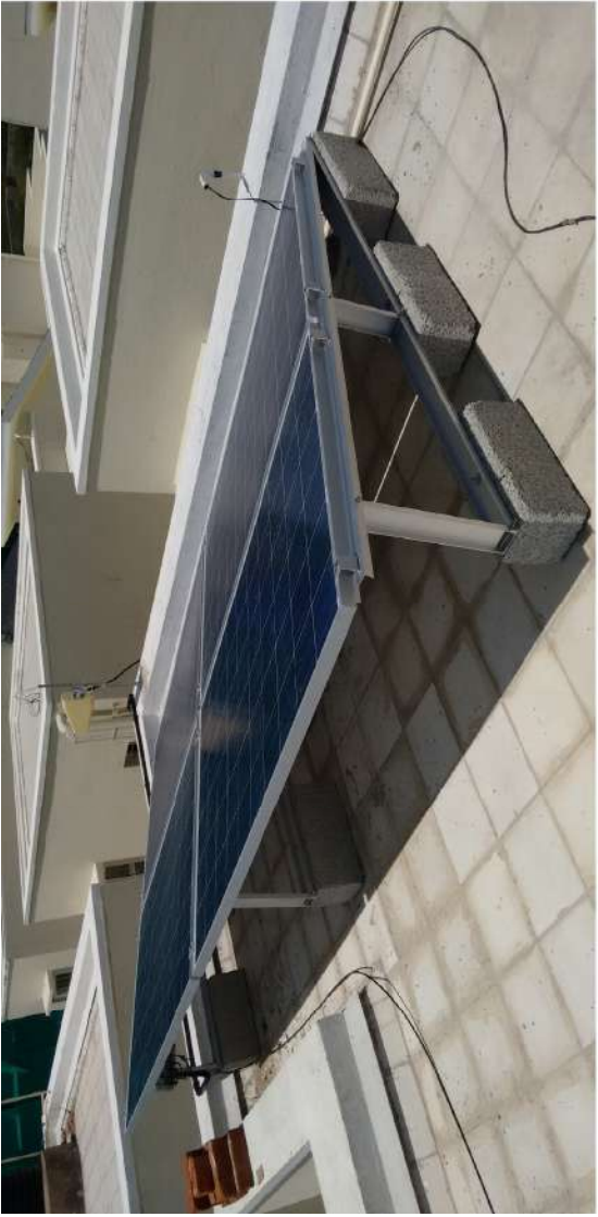
1KW Rooftop SPV Power Plant Installed at Perumbakkam, Chennai
