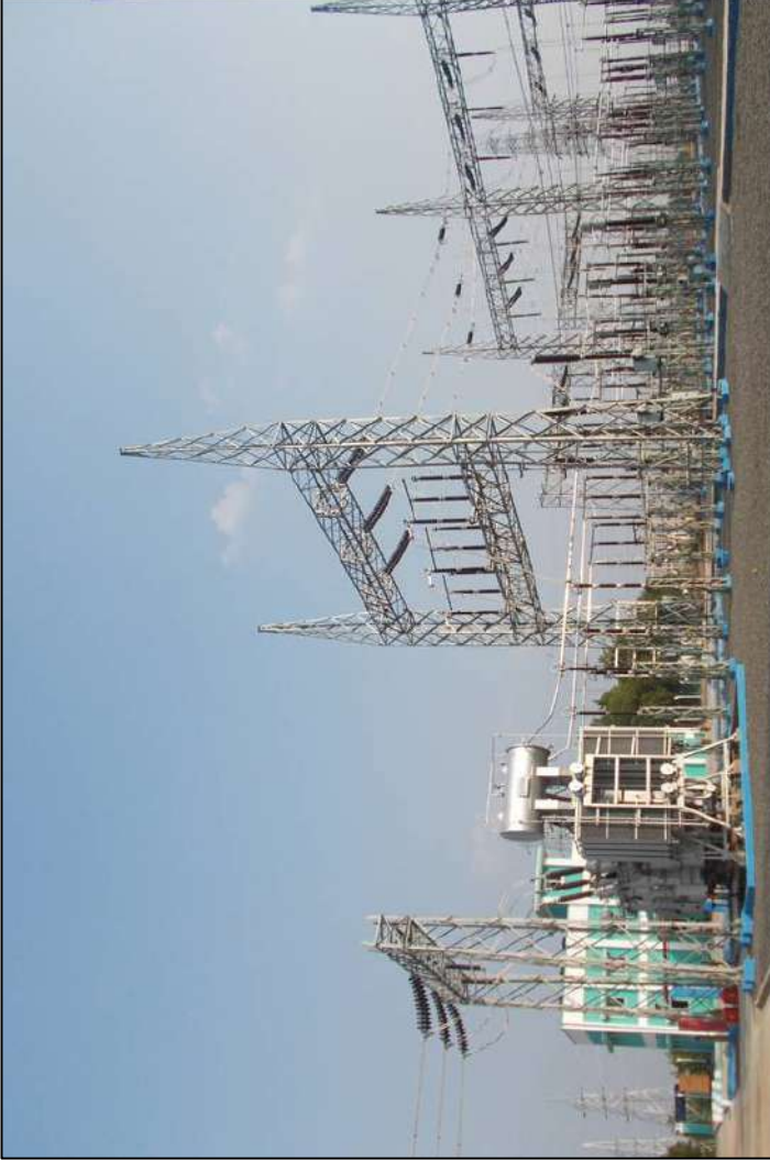
JICA scheme- Kinnimangalam 230/110kV substation – Madurai District
