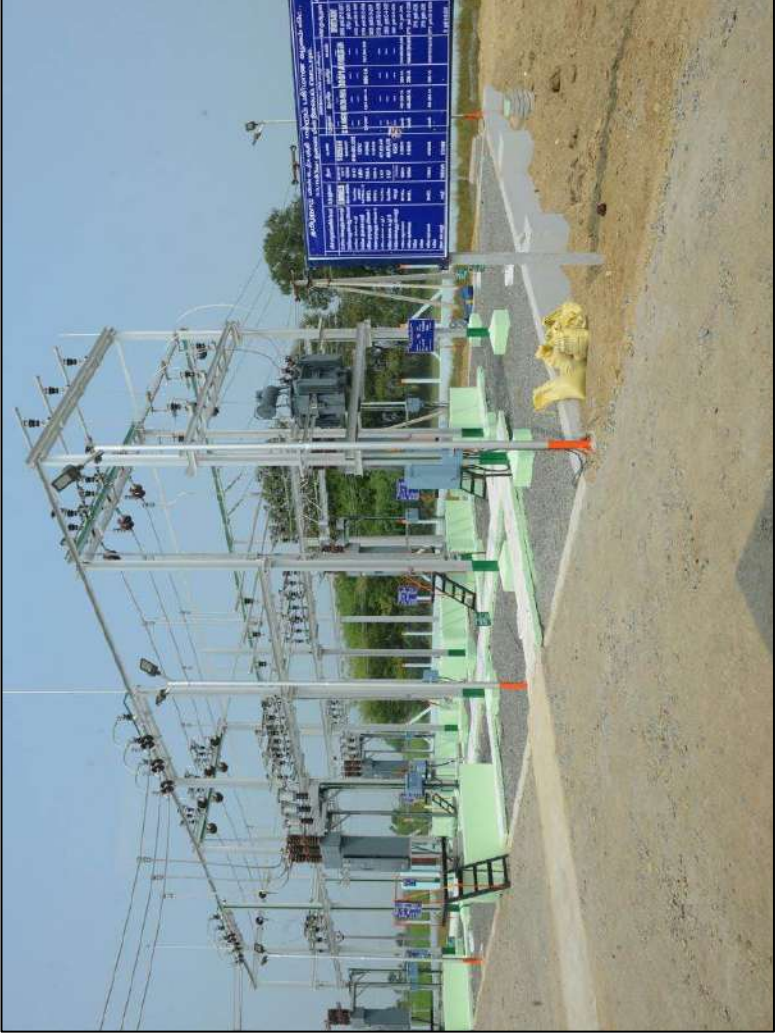
DDUGJY scheme- Kottaram 33/11 kV – Cuddalore District
