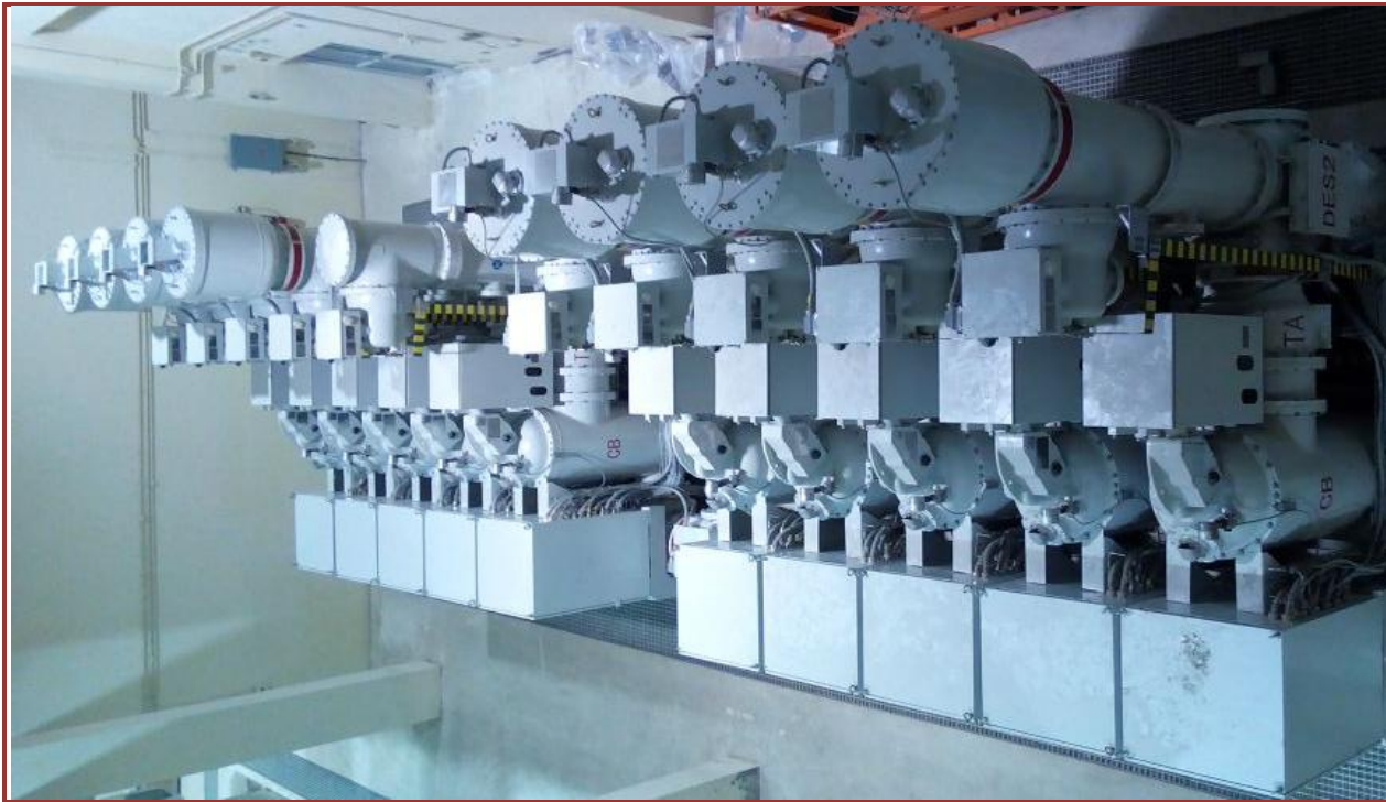
Alandur 230/110 - 33 kV GIS substation, Chennai
