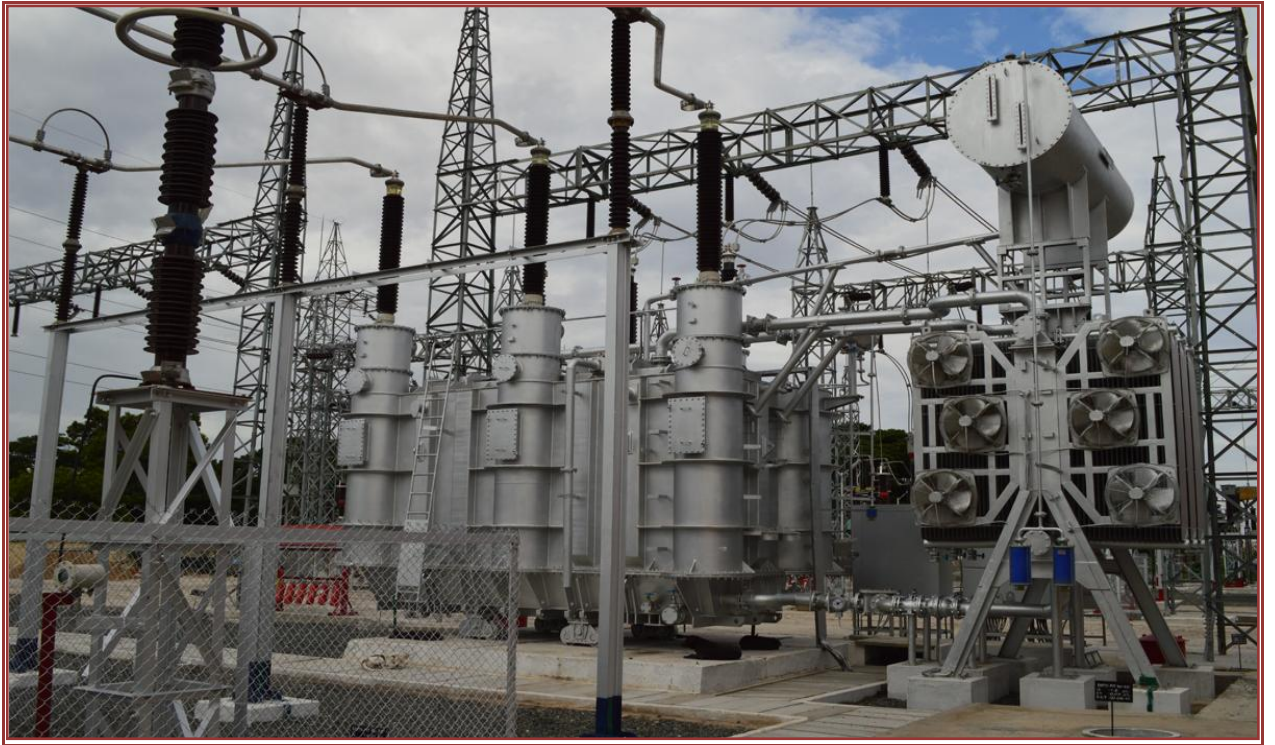
Coimbatore 230/110 kV Substation, Coimbatore District
