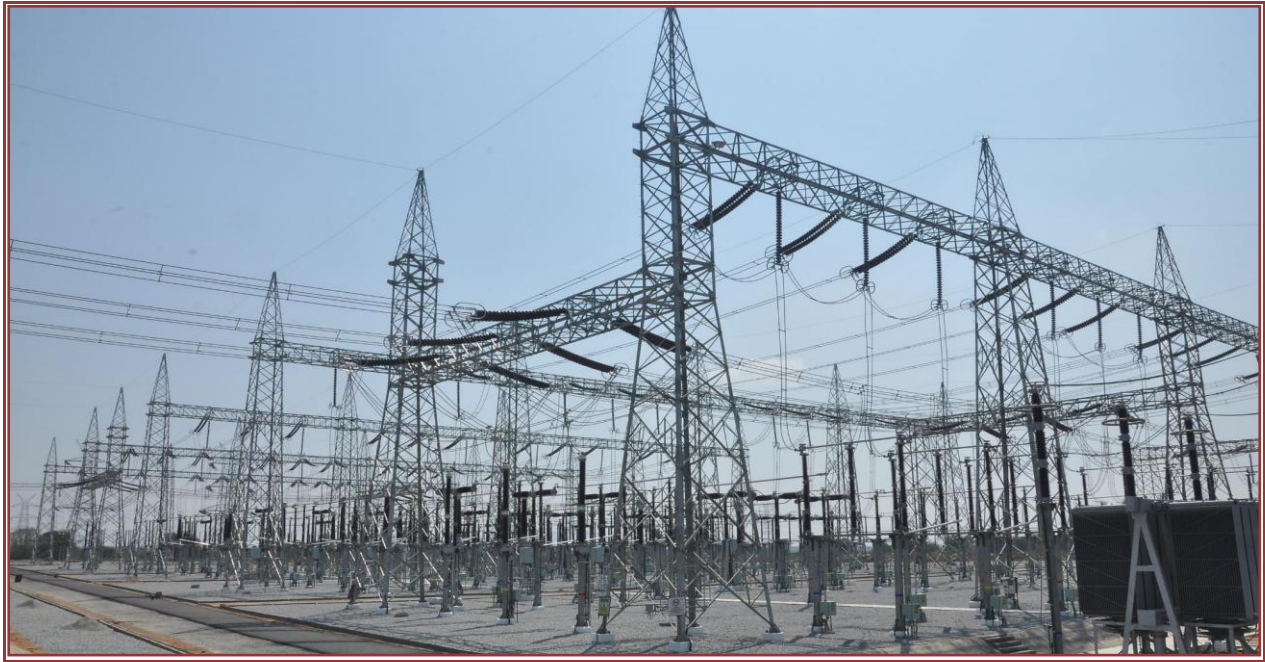
Tiruvalam 400 kV substation, Vellore District
