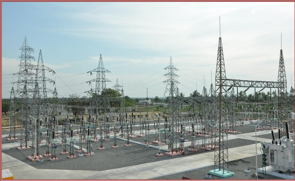
Anthiyur 230/110 kV substation, Erode District
