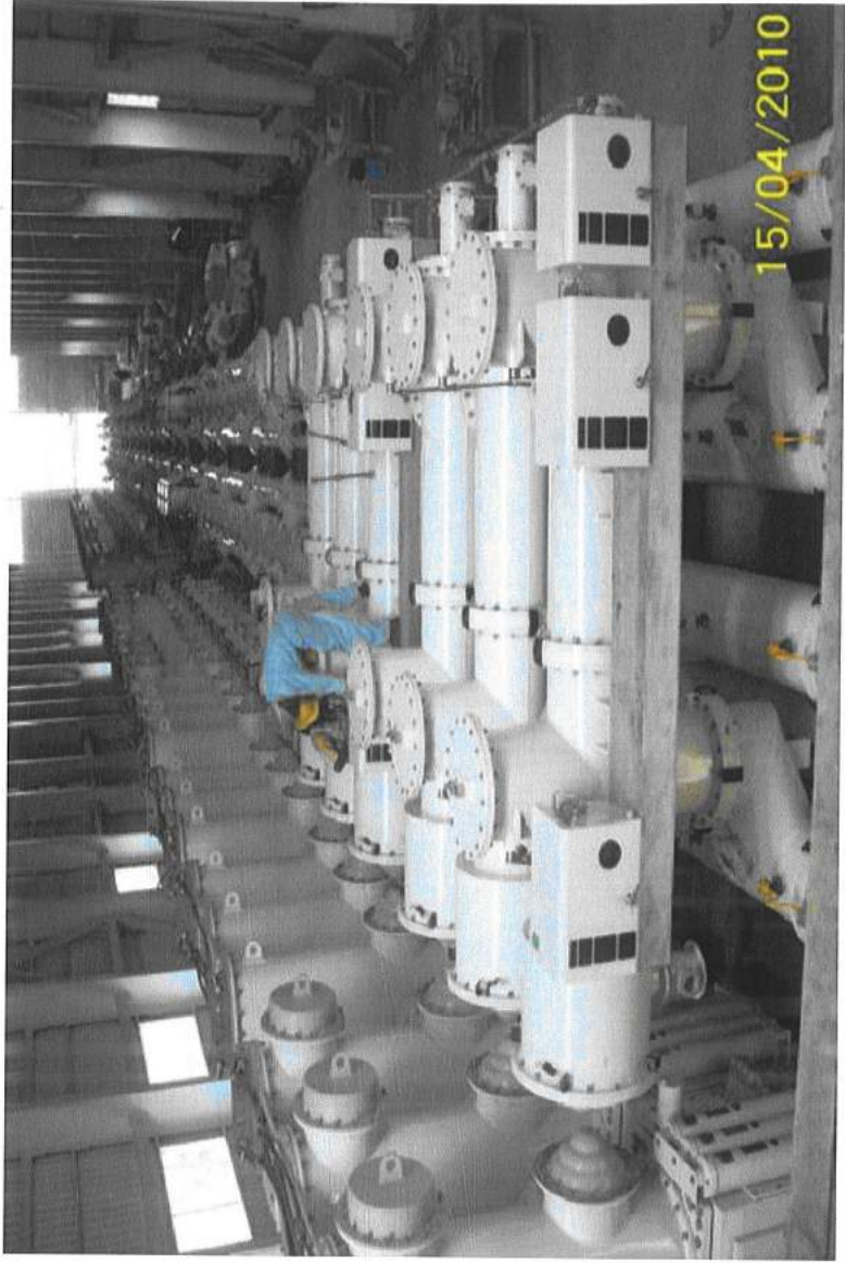
TNEB - NTPC JV PROJECT GIS- SWITCH YARD - VALLUR
