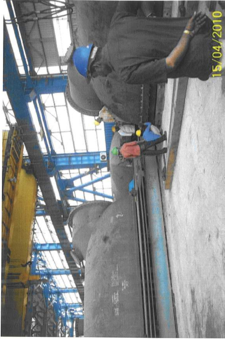
TNEB - NTPC JV PROJECT CONDENSOR WATER ASSEMBLY - VALLUR
