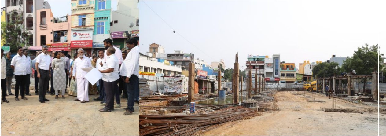
Hon'ble Minister for Hindu Religious and Charitable Endowments Department and Chairman CMDA inspected ongoing works of 2023 – 2024 announcement projects along with Department officials.
