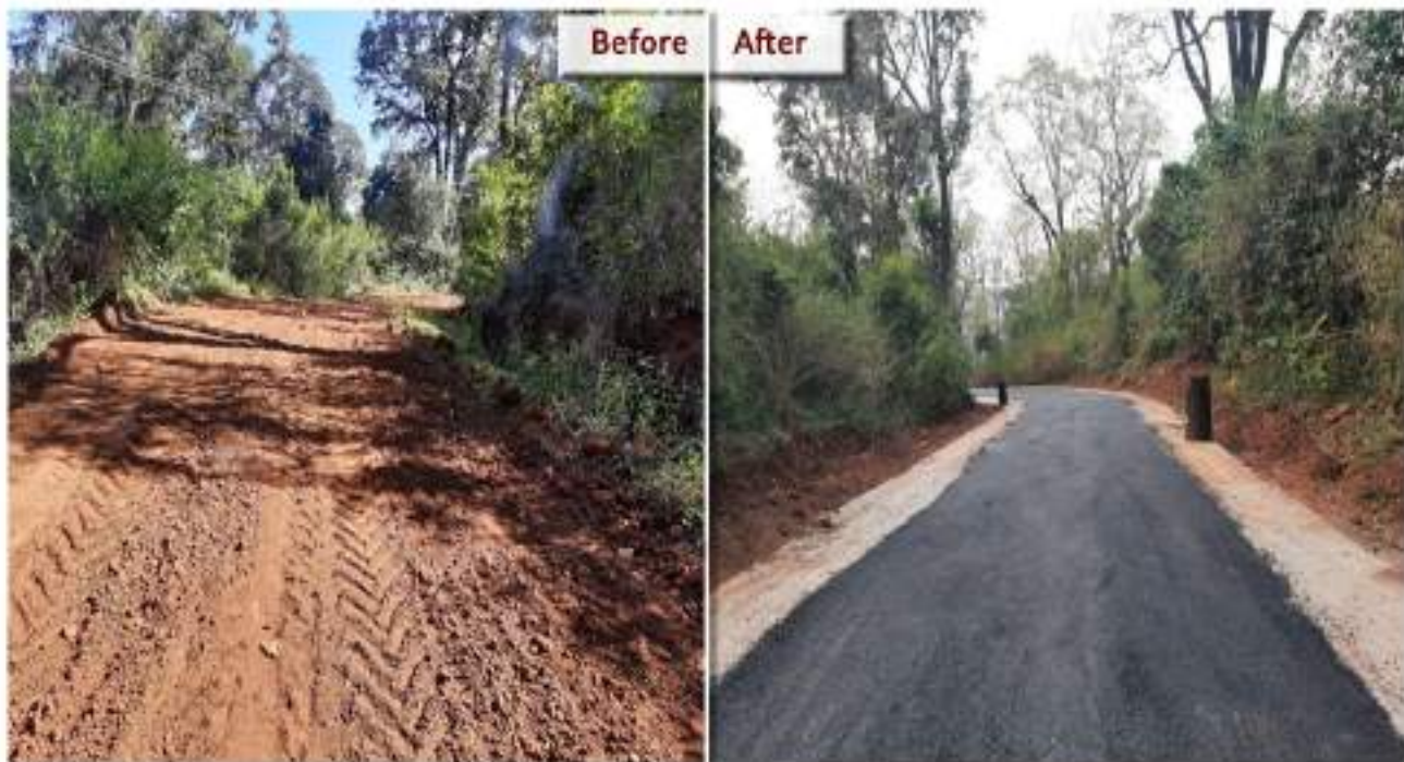
Namakkal District, Thirupulinadu to Keeraikadu Road work for Scheduled Tribes Habitations, (Estimate amount : Rs.60.50 lakh).
