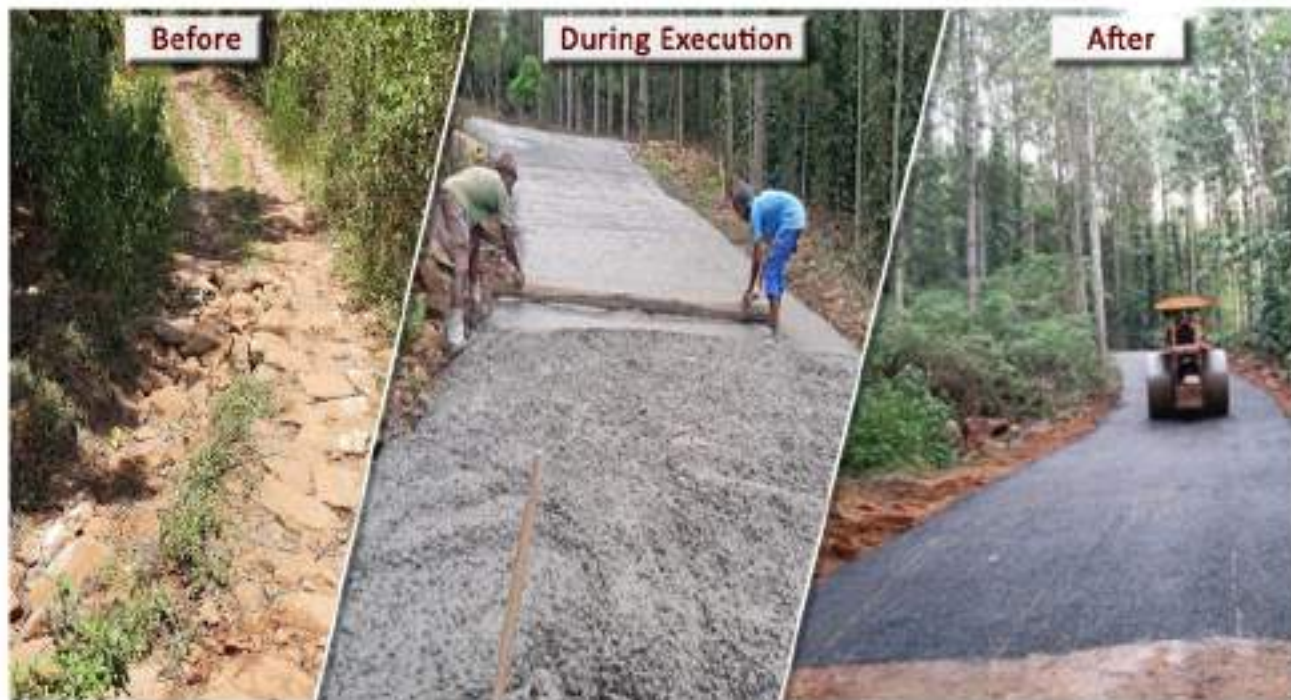
Salem District, Gundur to Kasikal Road work for Scheduled Tribes Habitations, (Estimate amount : Rs.110.00 lakh).
