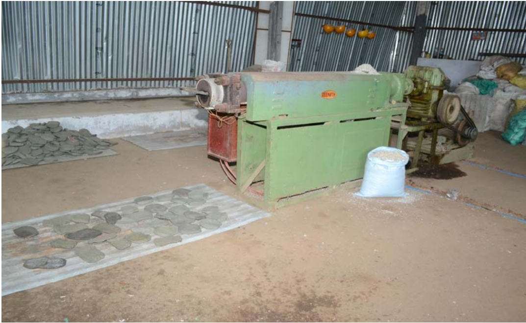
Plastic waste recycling unit at Thudiyalur Town Panchayat.
